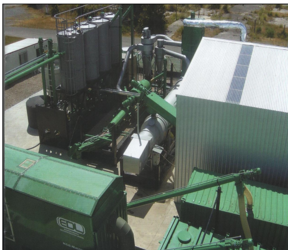
MCD process at the Mapua Site. Source: Ref. 54
