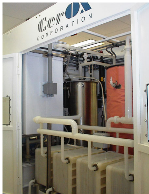
CerOx™ treatment system, Source: Ref. 9
