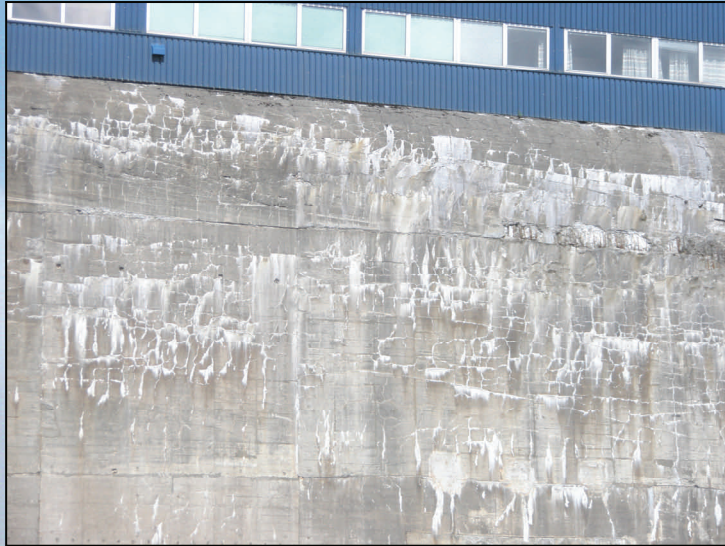
Wall built with ASR susceptible aggregate showing ASR gel extruding from the cracks. (Photo taken during the 13th ICAAR field trial trip in Norway, submitted by Gina Ahlstrom)
