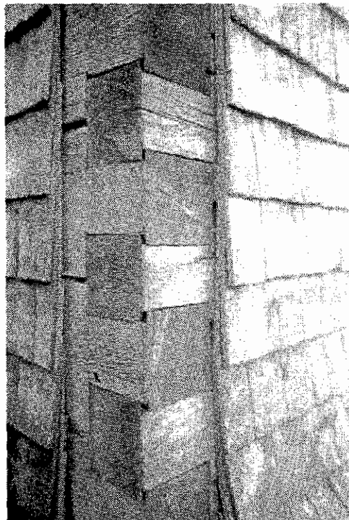
Figure 4.78. Corner notching detail, Lars Christian Alstrom / Peter Stormer house ruin, 1996. Although the Peter Stormer family abandoned the house more than seventy years ago, all four of its side walls remain standing and remarkably intact. Such longevity attests to the durability of the solid corner-joints and exquisite craftsmanship that are evident in the wall construction.
