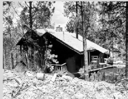
The McDonald home had only minor exterior damage. Homes on both sides were completely destroyed by flames.
