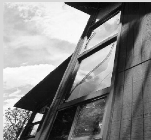
The McDonalds credit the use of double-paned windows as one of the construction barriers that prevented the fire from entering their home. The outer layer absorbed the fire's force and shattered.
