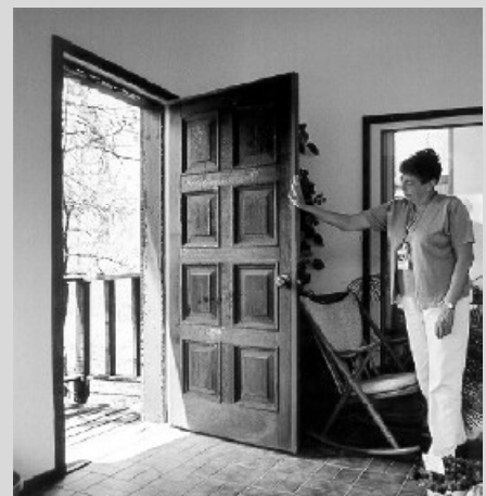
Myrna McDonald holds open the severely singed solid core door that prevented flames from entering the interior.
