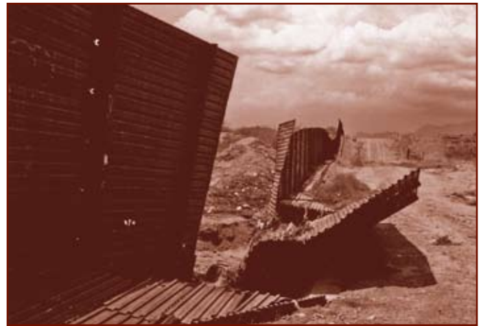
Installation of security fencing without regard for environmental factors such as stormwater runoff may produce accelerated erosion and resulting instability. (Source: International Boundary and Water Commission)
