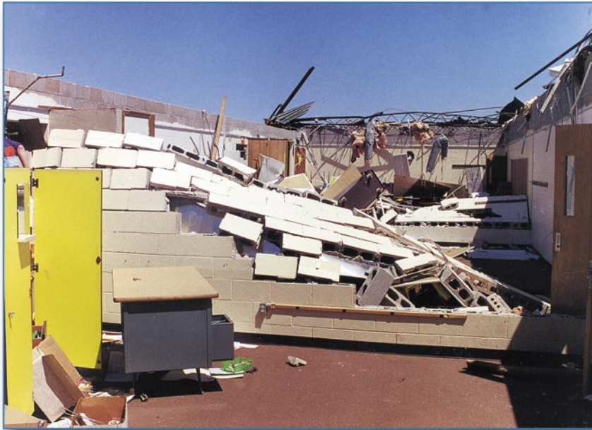
Figure 6-34 The interior walls of this classroom wing were constructed of unreinforced CMU.
