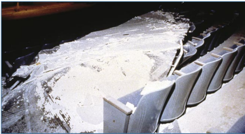
Figure 4-13 Fallen heavy lath and plaster ceiling across auditorium seating, Northridge, CA, 1994 SOURCE: GARY MCGAVIN, REDLANDS, CA
