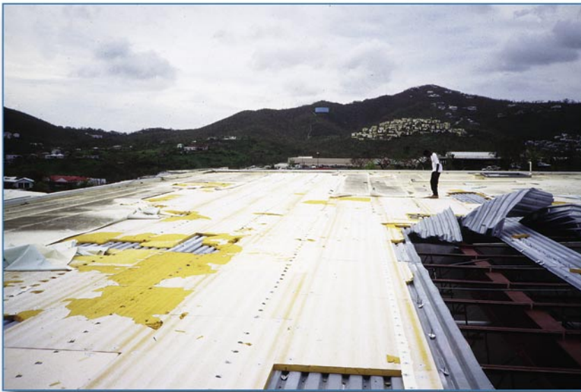
Figure 6-41 On this school, the fastener rows of the mechanically attached single-ply membrane ran parallel to the top flange of the steel deck. Hence, essentially all of the row's uplift load was transmitted to only two deck fasteners at each joist (as illustrated in Figure 6-42). Because the deck fasteners were overstressed, a portion of the deck blew off and the membrane progressively tore.
