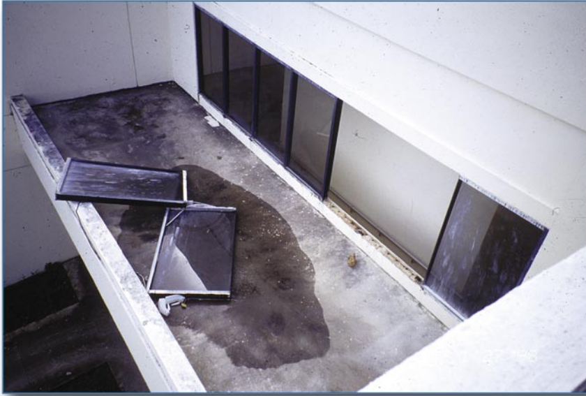
Figure 6-45 Two complete windows, including their frames, blew out. The frames were attached with an inadequate number of fasteners, which were somewhat corroded.
