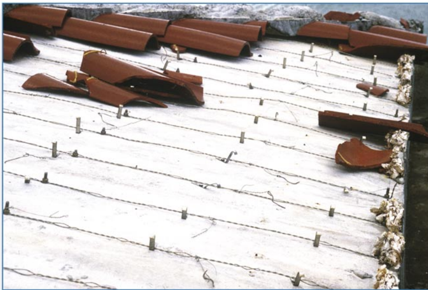
Figure 6-52 These wire-tied tiles were installed over a concrete deck. They were attached with stainless steel clips at the perimeter rows and all of the tiles had tail hooks. Adhesive was also used between the tail and head of the tiles.
