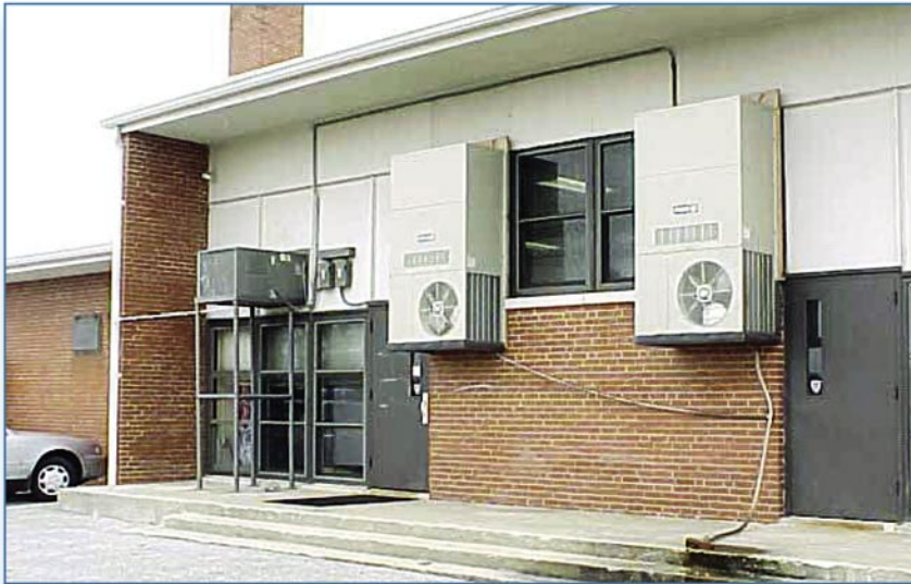
Figure 5-14 Elevated utilities behind an elementary school in Wrightsville Beach, NC
