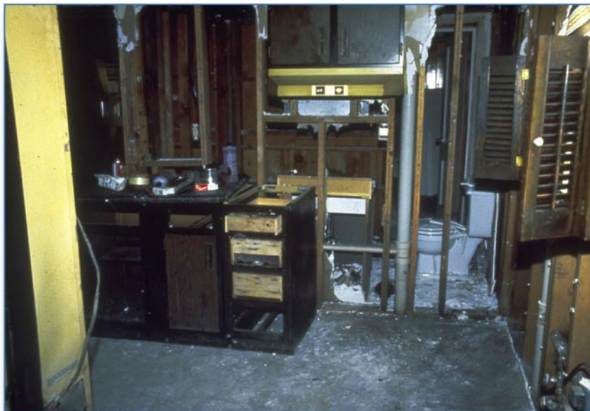
Figure 5-9 Damaged walls and cabinets, Peoria County, IL
