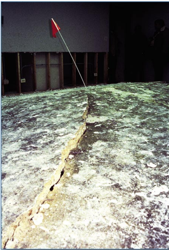
Figure 5-8 Fractured concrete basement floor, Gurnee, IL, 1986
