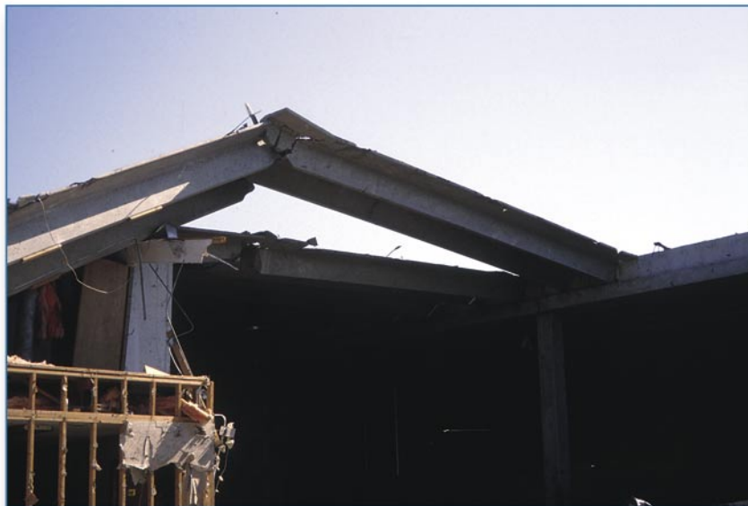
Figure 6-24 Several of the precast twin-Tee roof and wall panels collapsed. The connection between the roof and wall panels provided very little uplift load resistance. This roof panel lifted because of combined effects of wind uplift and pretension.
