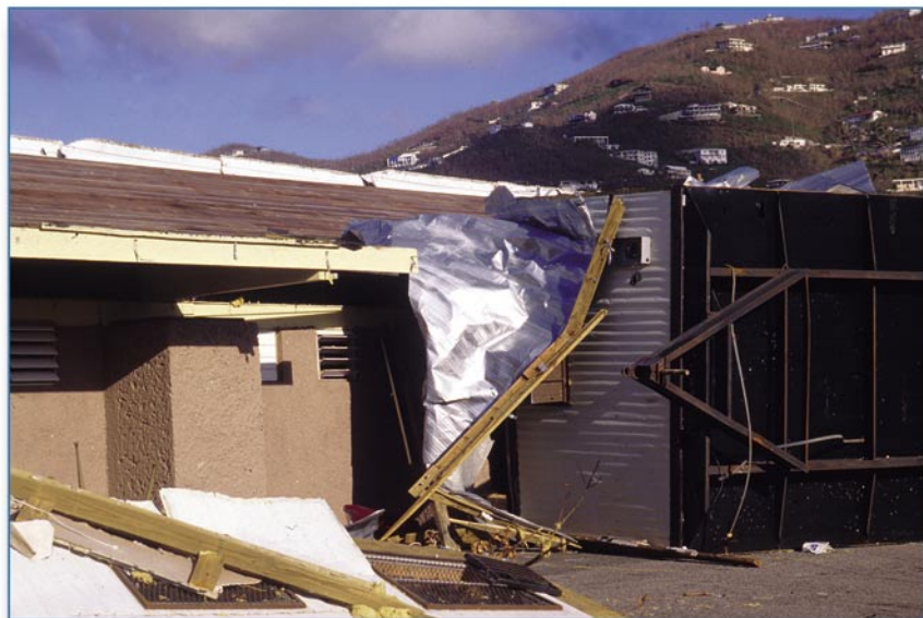
Figure 6-16 This portable classroom was blown up against the main school building during a storm that had wind speeds that were less than the design wind speed. Depending upon the type of exterior wall, an impacting portable classroom may or may not cause wall collapse.
