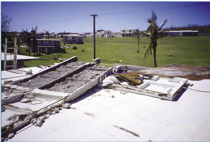
Figure 6-23 Portions of this waffled precast concrete roof deck were blown off. Bolts had been installed to provide uplift resistance; however, anchor plates and nuts had not been installed. Without the anchor plates, the dead load of the deck was inadequate to resist the wind uplift load.
