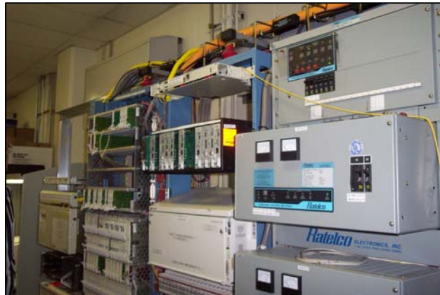
Figure 14. Telecom and Network Connections
