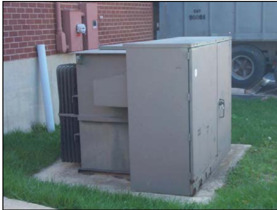
Figure 18. One of Two Transformers On Site
