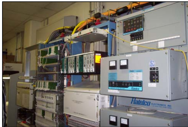
Figure 23. Telecom and Network Connections
