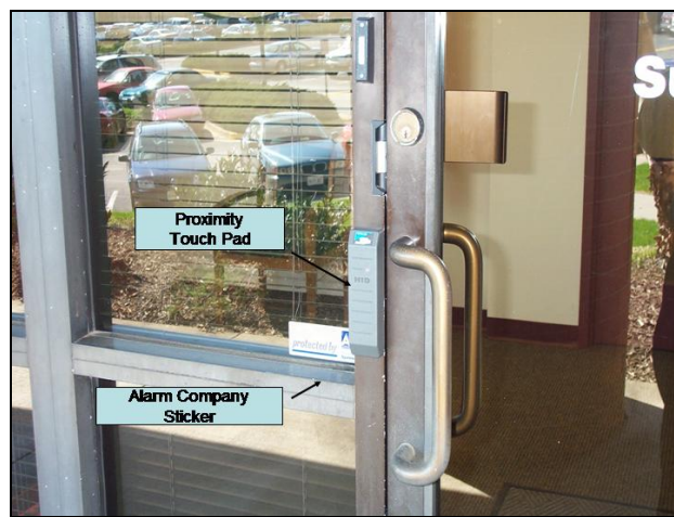
Figure 25. Proximity Card Readers and Alarms
