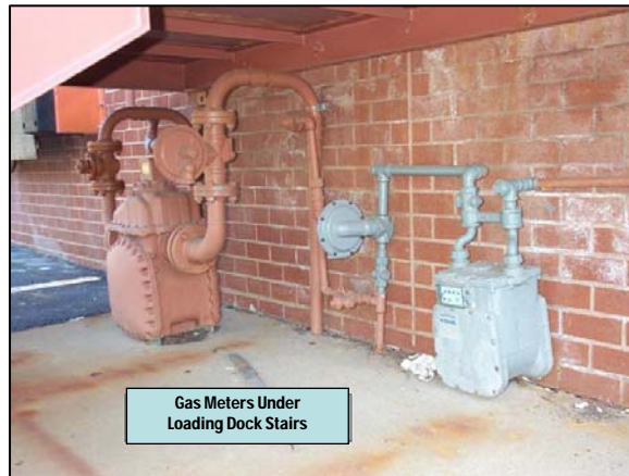
Figure 16. Gas Meters Under Loading Dock Stairs
