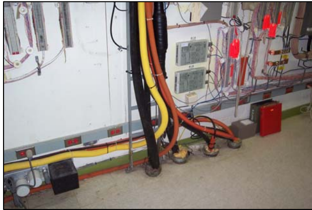
Figure 22. Telecom and Network Connections
