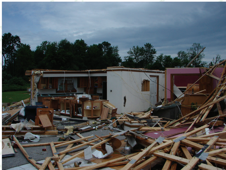
Above: This home in Rush county was severely damaged by EF3 tornado winds.
