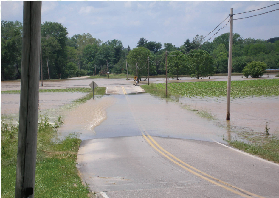
Above: Water flows over a road near Columbus IN. Driving through flood waters is extremely dangerous. Turn around, Don't Drown!
