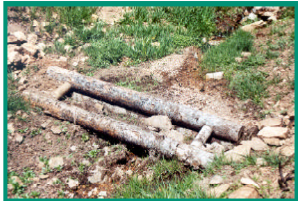
One of the flow check structures installed on a burned over slope.
