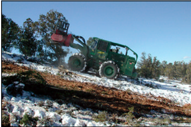
The environmental brush cutter working on the Joel Spring Project during the winter months.
