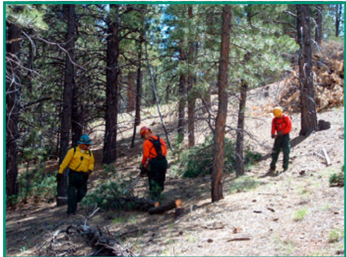
Mammoth Creek defensible fire space zone on the south side. Crews thinning and piling.
