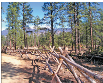
Buck and rail fence build from thinned poles by an inmate crew.
