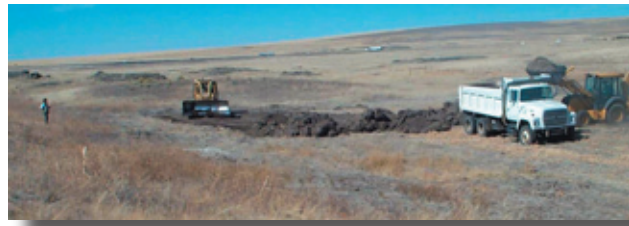
The Turnbull National Wildlife Refuge heavy equipment crew scalps away the sod because it contains seed and rhizomes that would re-invade the wetland.
