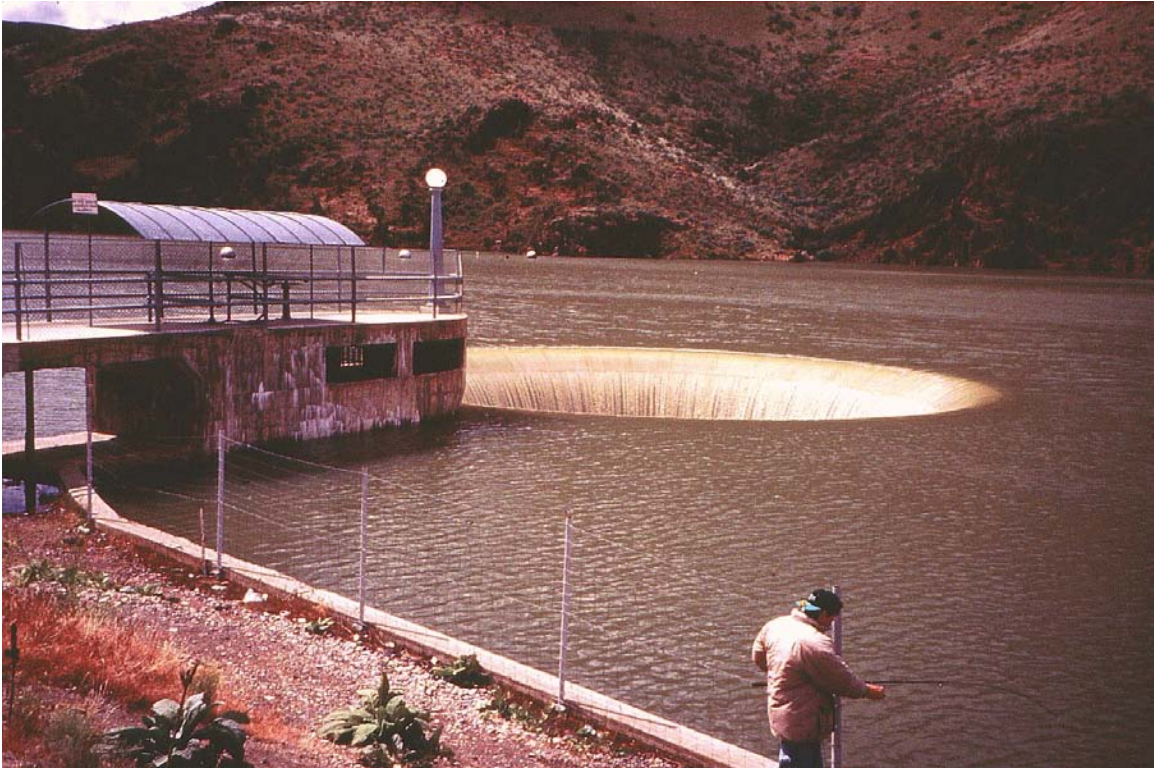
Figure 1c.—The movable ring gate outlet behind the dam on the right abutment seen in Spring 1996.
