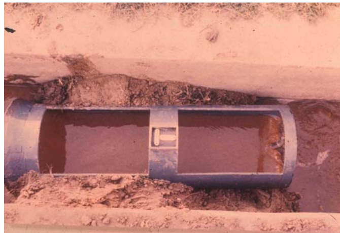
Figure 10. — Portable Flume Constructed in a Section of Circular Pipe.
