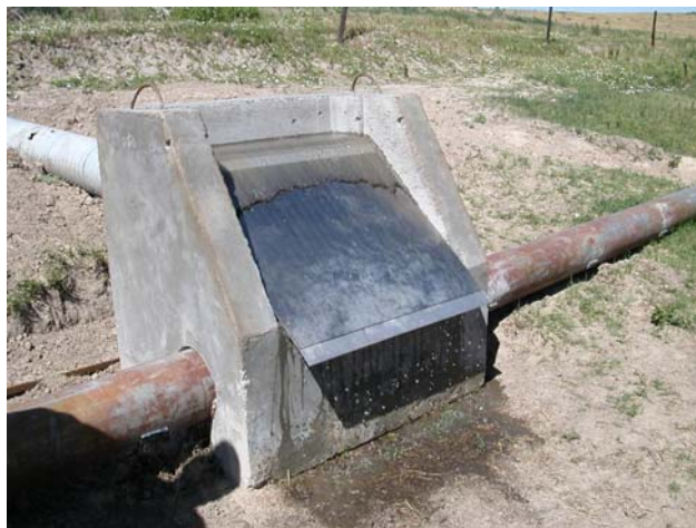
Figure 4. — Coanda-effect screen structure feeding two irrigation pipelines. Raw water enters the back of the structure through the white, PVC pipe. Screened water exits to the right and left. Overflow and debris are discharged onto the ground at the front of the screen.
