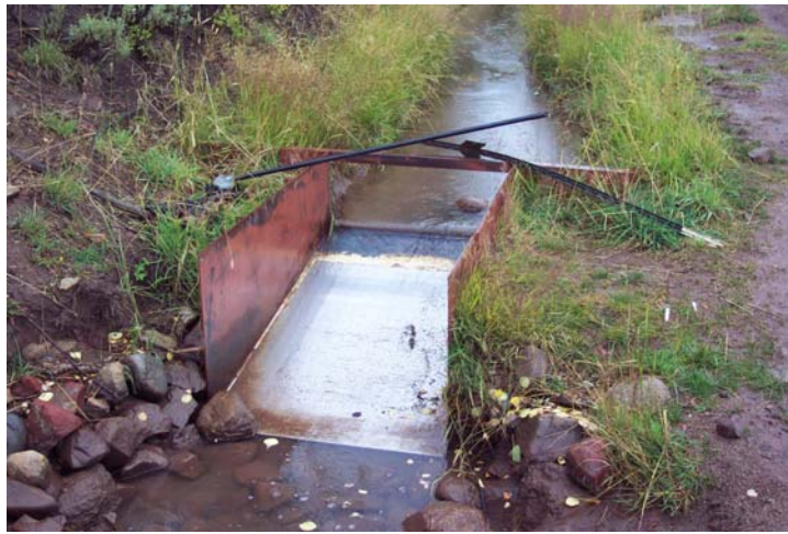
Figure 11. — A small Coanda-effect screen provides water to a sprinkler irrigation system near Carbondale, Colorado.
