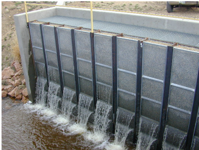
Figure 6. — Sand filter at Lake John. This structure presented some exciting maintenance challenges.
