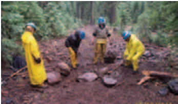
Civilian Conservation Corp crews working on the Pacific Crest Trail on the Almanor Ranger District
