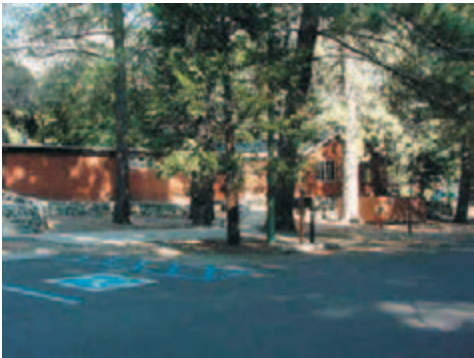
Adventure Pass funds were used to repair this parking lot at the Mt. Baldy Visitor Center.
