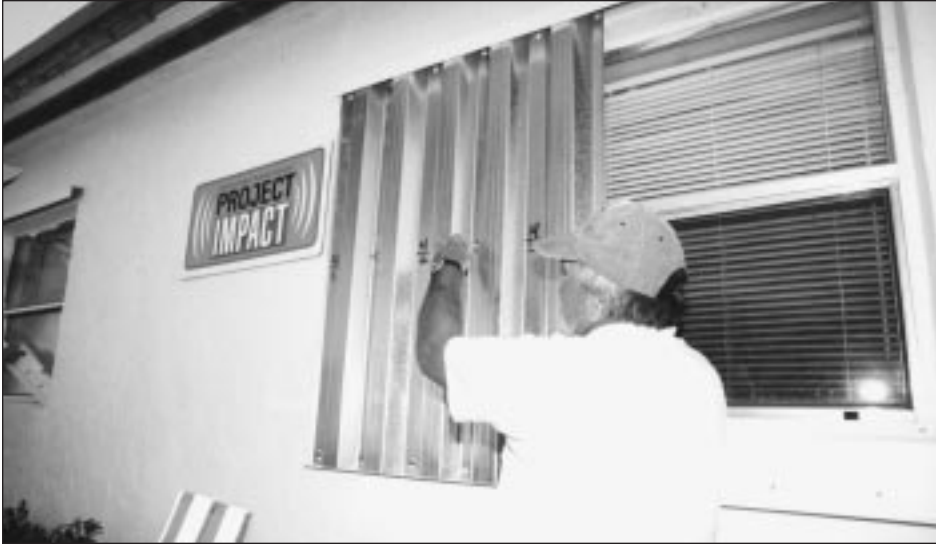
A Deerfield Beach resident installs hurricane shutters as part of that community's active participation in Project Impact.
