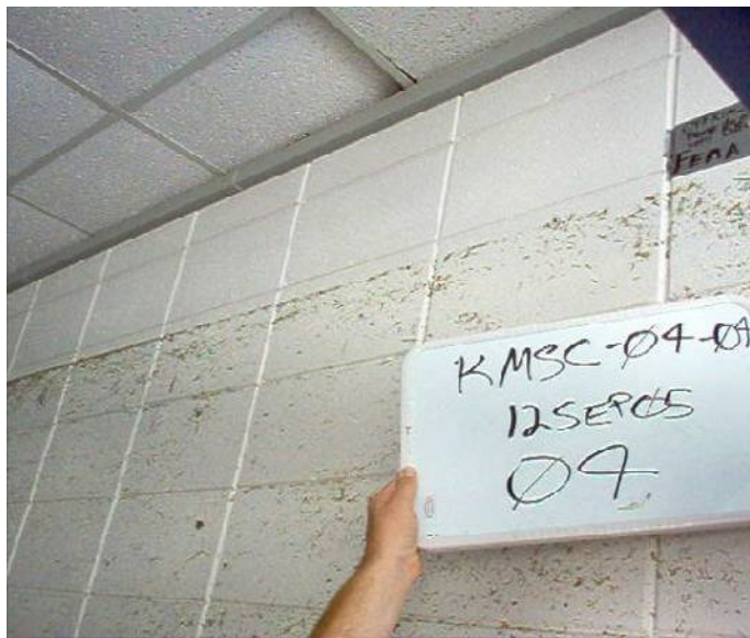
Figure 6 – Interior Mud Line HWM
