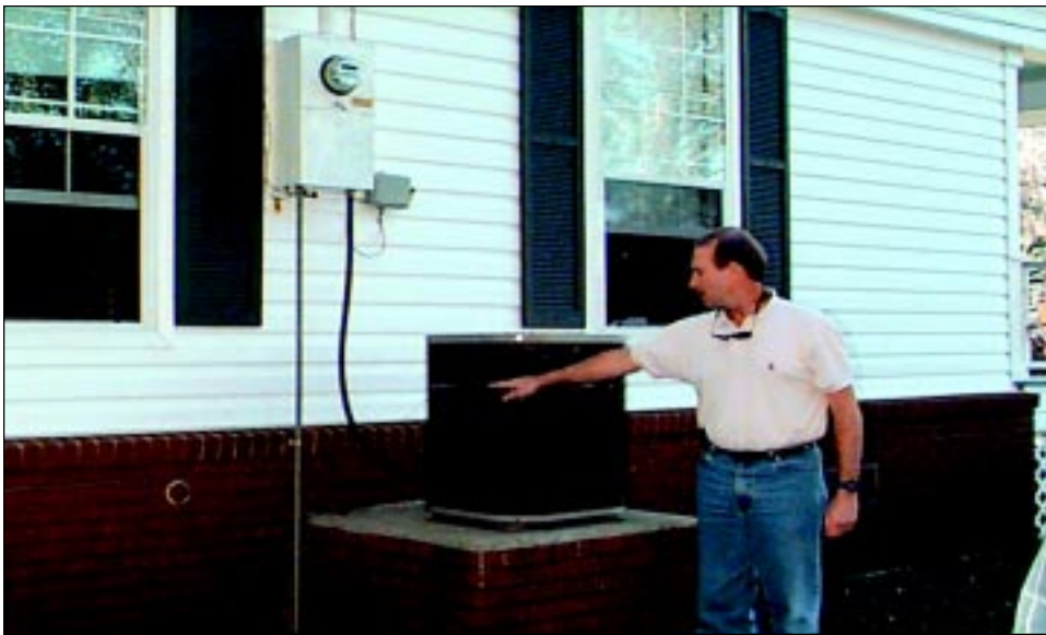
FIGURE 6-5 The high water mark on the air conditioner compressor indicates that the flood level was approximately 3 inches above the lowest floor.
