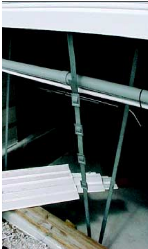
FIGURE 5-24 Improper strap installation. The buckle should be positioned where the strap wraps around the beam as shown in Figure 5-25.
