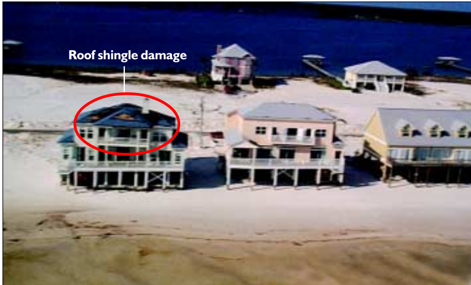
FIGURE 5-13 The house on the left suffered wind damage to roofing shingles.
