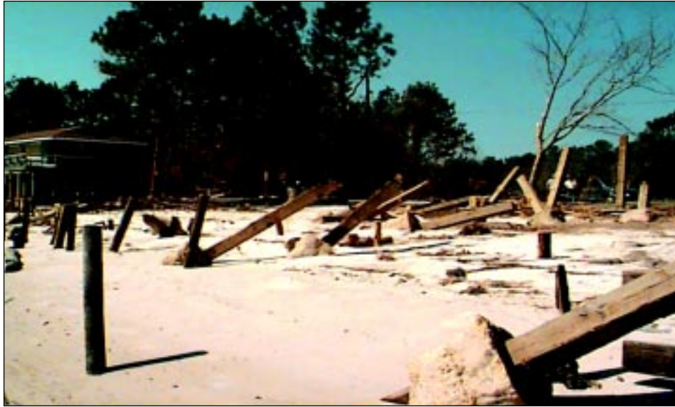
FIGURE 6-14 The houses in this area were destroyed. Piles were embedded in concrete to a depth of only 2 feet. Storm-induced erosion of 2 to 3 feet resulted in complete failure of the foundation systems.
