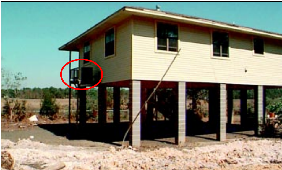
FIGURE 6-17 This house was set back 100 feet or more from the open coast out of reach of velocity flow and wave action. Note elevated utility platform.
