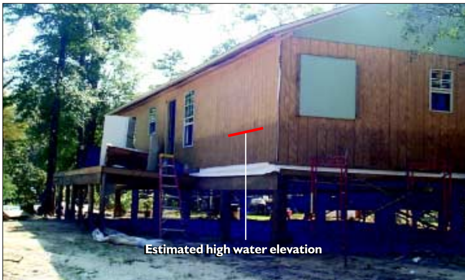
FIGURE 5-2 A high water mark is visible approximately 3 feet above the first floor elevation. The house, located along the Shoal River in Okaloosa County, suffered little damage because insulation and wallboard had not yet been installed.
