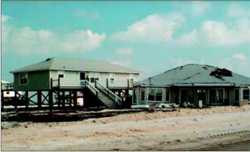
FIGURE 4-10 The structure on the right lost its pile foundation system and was washed into the structure on the left.
