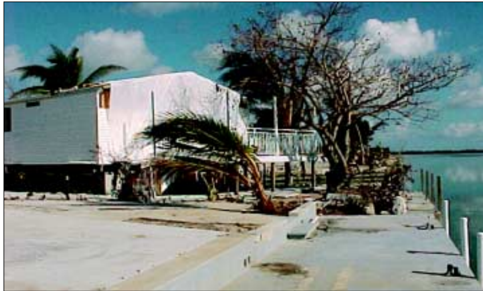
FIGURE 5-17 This home suffered damage when its awning blew off. The lot next door contained an older manufactured home that was completely destroyed by high winds and coastal surge.
