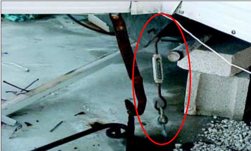
FIGURE 5-22 Inadequate turnbuckle anchor installed by homeowner on this older manufactured home. The home was severely damaged due to the lack of elevation, an unreinforced foundation system, and poor anchoring.
