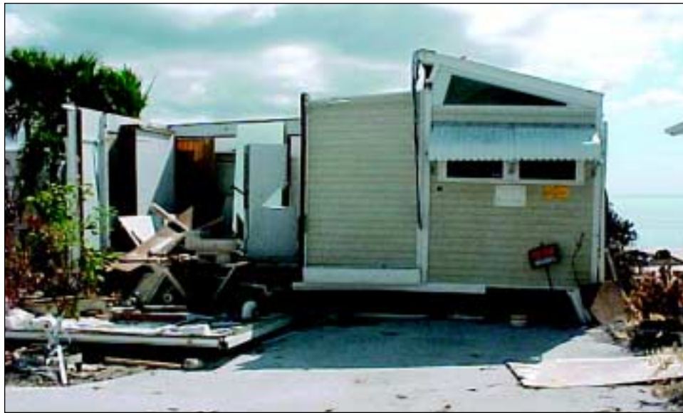
FIGURE 5-20 Older, non-elevated manufactured home with an addition that sustained substantial damage.
