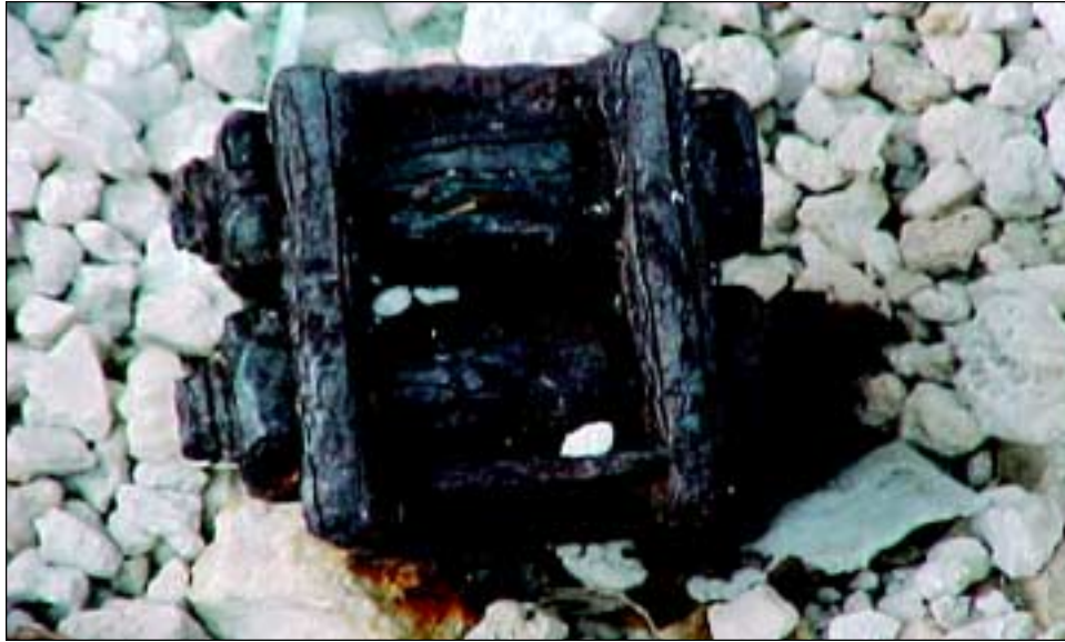
FIGURE 5-23 Rusted anchor under an older manufactured home. The State of Florida mandated galvanized anchors after January 1, 1999.
