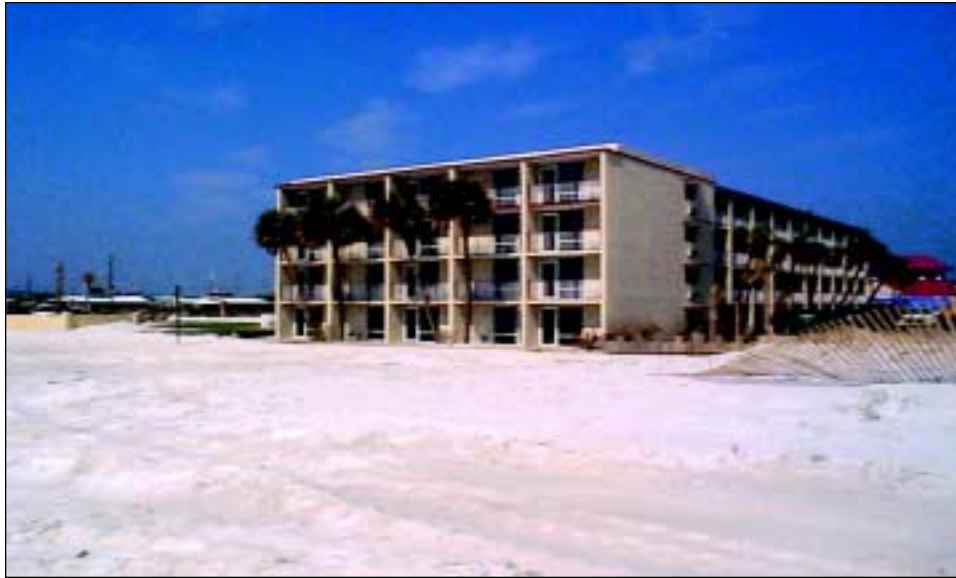
FIGURE 5-11 An older hotel that suffered significant damage to the interior due to storm surge and roof leakage.
