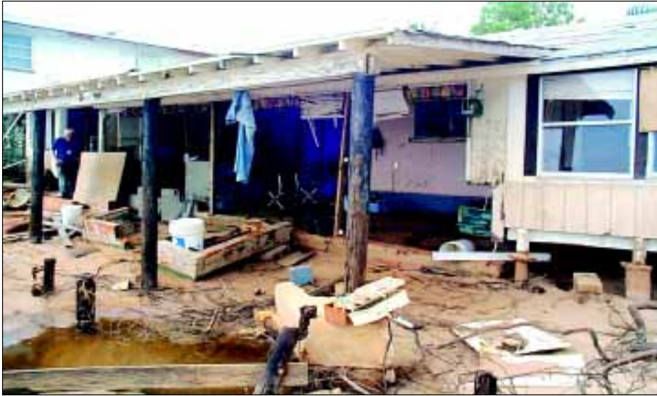
FIGURE 4-31 Non-elevated pre-FIRM structure severely damaged by coastal storm surge.
