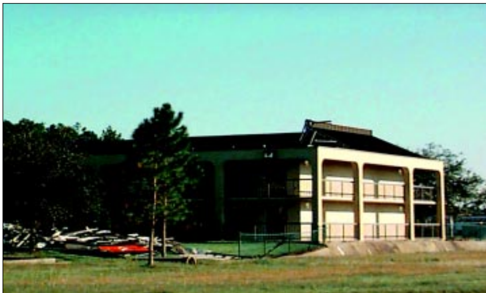
FIGURE 6-20 Roof damage to a hotel in Pascagoula.
