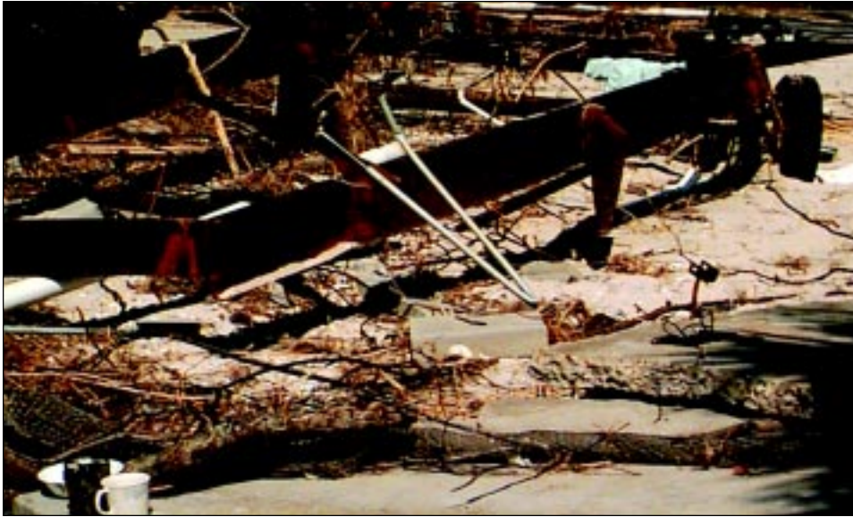
FIGURE 6-16 All that remains of this oceanfront manufactured home that was located on this lot is the bent metal frame. The foundation system was dry-stacked blocks. Tiedown anchors on the Gulf side of the home failed due to erosion and flood forces.
