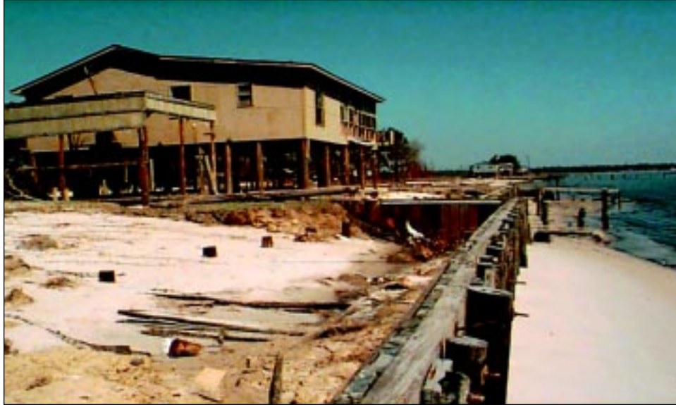
FIGURE 6-10 Scour behind bulkhead near Belle Fontaine.
