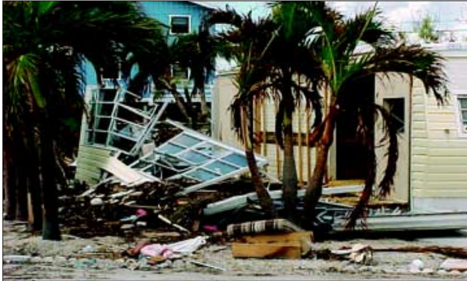
FIGURE 5-26 The addition to this manufactured home was destroyed, causing considerable damage to the rest of the home.
