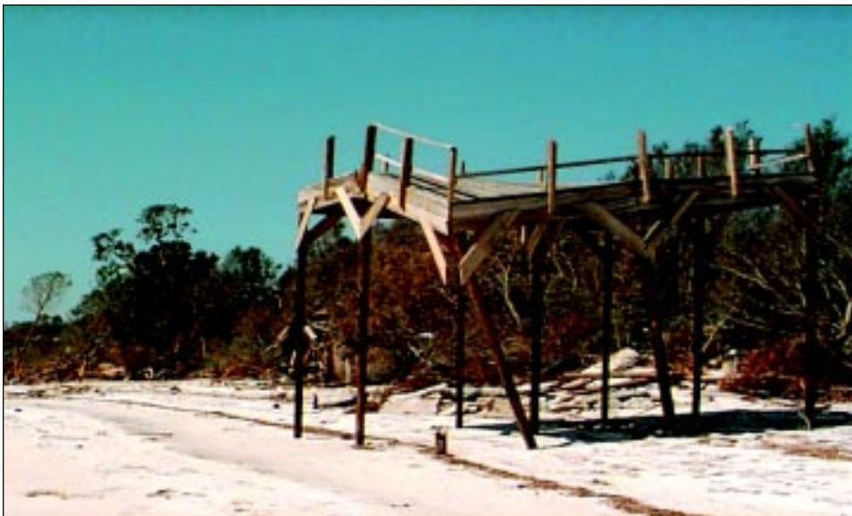
FIGURE 6-13 Only the deck remains standing on this home. House debris can be seen in the background. Storm-induced beach erosion and inadequate pile embedments contributed to the failure of this home.
