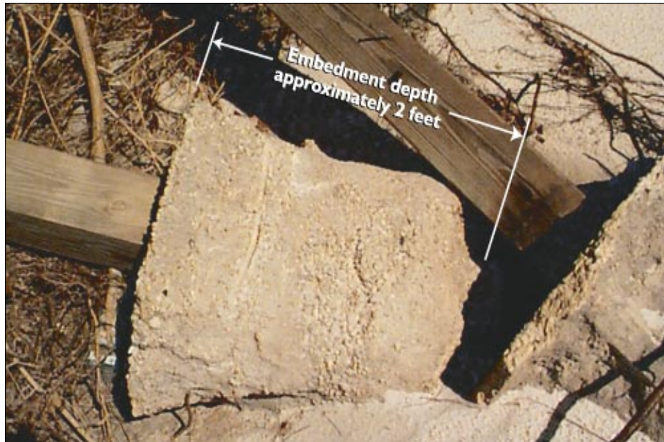
FIGURE 6-15 Inadequate embedment of piles from a destroyed home.
