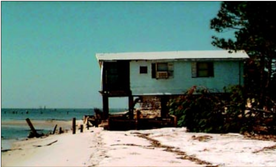
FIGURE 6-12 Highly exposed structure that suffered damage from storm surge and high winds.
