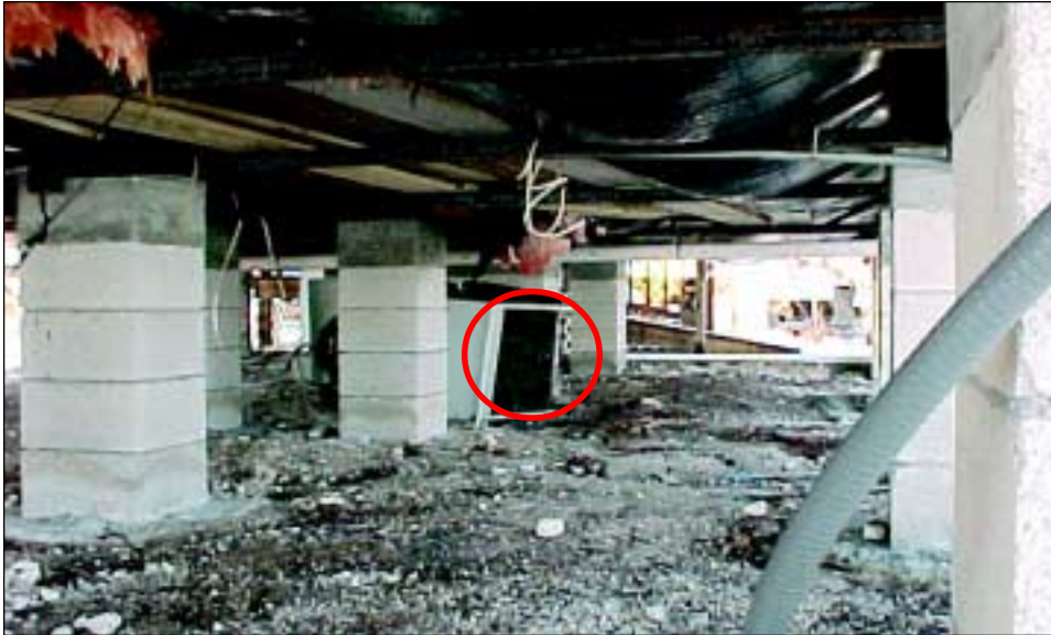
FIGURE 5-18 Reinforced masonry pier foundation system under a newer manufactured home that performed well. The air conditioner compressor (circled) washed under the home provides evidence of the coastal surge at this location.
