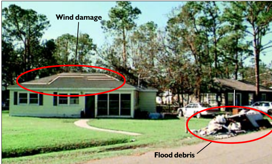
FIGURE 6-1 Home in Pascagoula that sustained wind and flood damage.
