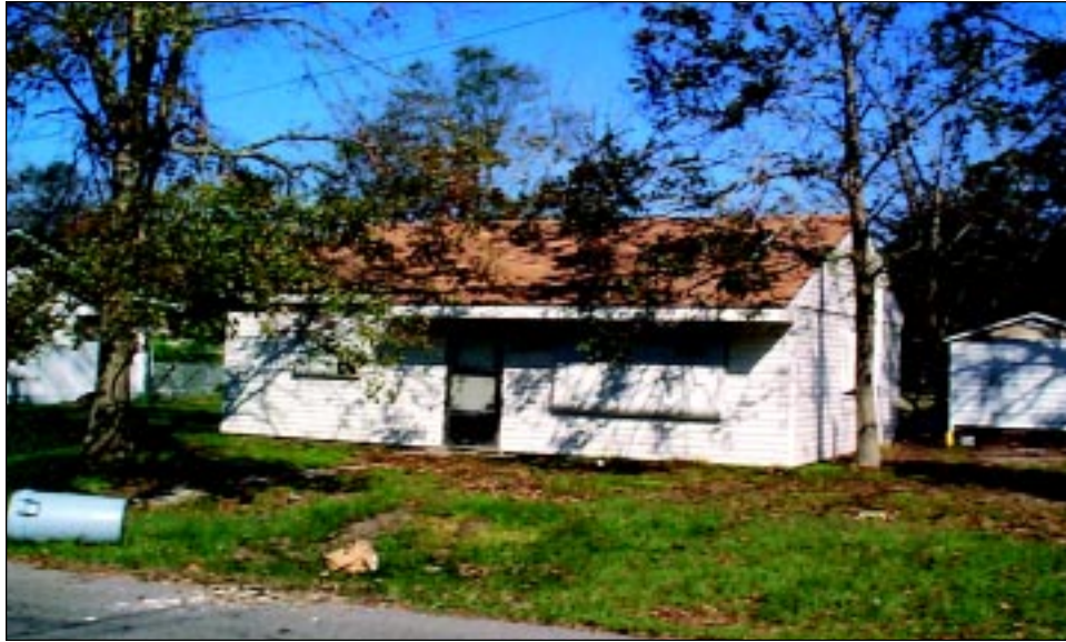
FIGURE 6-3 This home has suffered flood damage on numerous occasions. During Hurricane Georges it flooded several feet.
