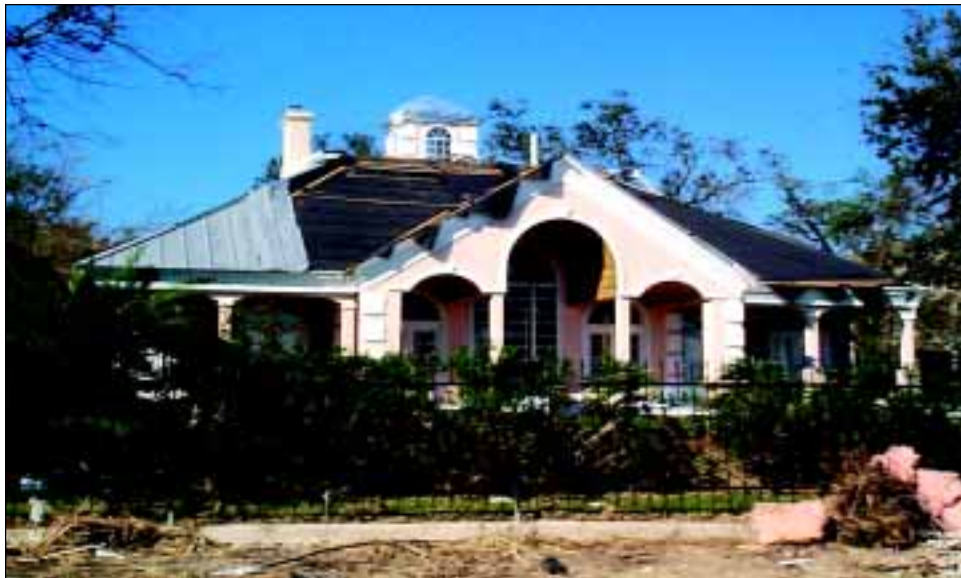
FIGURE 3-12 Wind damage to roofs and trees in Pascagoula, Mississippi.
