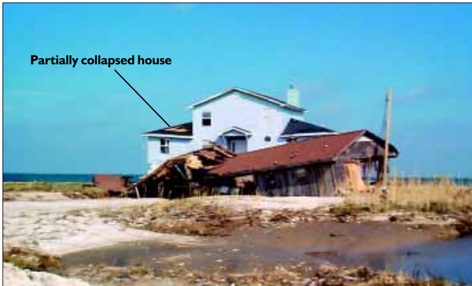
FIGURE 4-16 House on back side of Dauphin Island suffered partial collapse when impacted by a dislodged house from the Gulf side of Dauphin Island.
