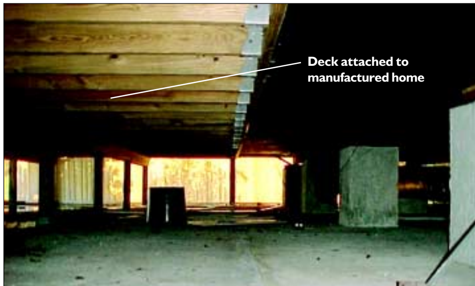
FIGURE 5-27 The underside of a deck that has been attached to the sidewall of a new manufactured home. The deck is not anchored as well as the home.
