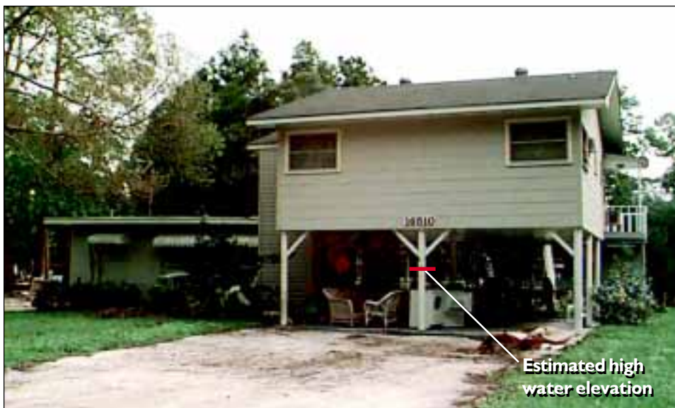
FIGURE 4-2 Approximately 5 feet of flooding at this house along the Fish River caused no damage to the elevated addition.
