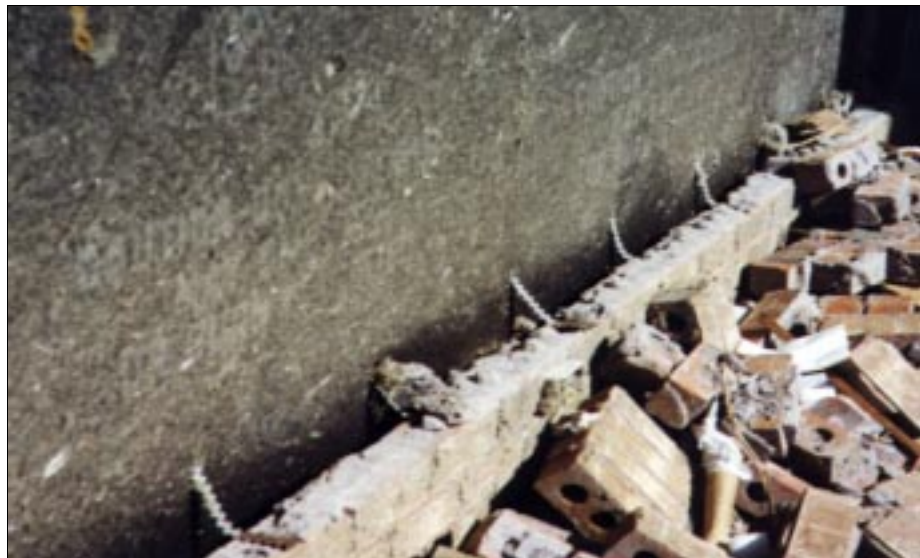
FIGURE 4-33: Failure of masonry veneer wall, close-up view, Moore, Oklahoma. This home was located along the periphery of a violent tornado.
