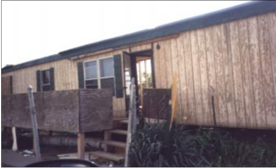
Figure 4-55: Damage to a manufactured home located on the periphery of a severe tornado, Wichita, Kansas.
