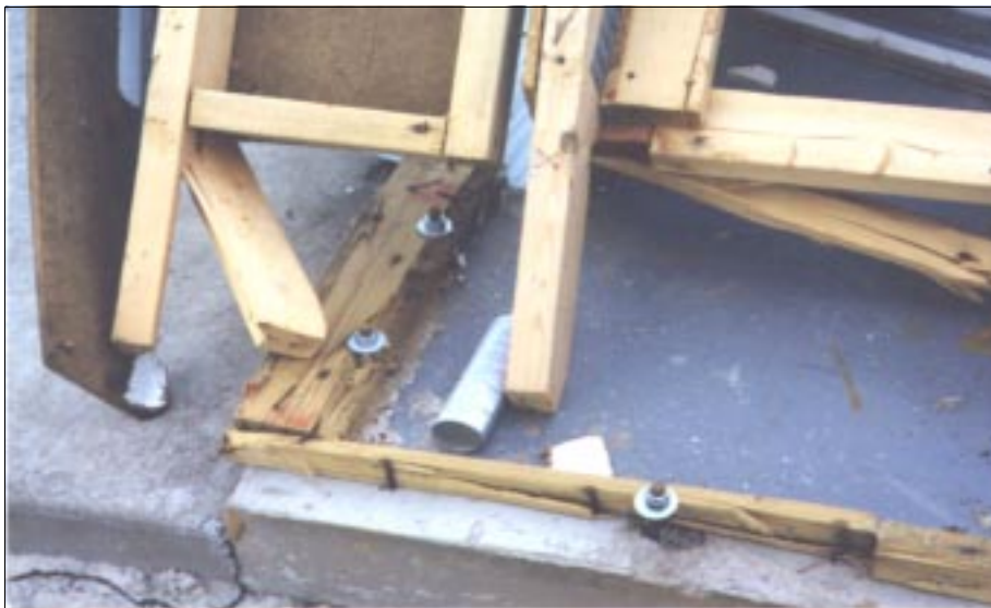
FIGURE 4-12: Failure at base of wall between wall studs and sill-plate. The sill-plate, which was connected to the foundation slab with anchor bolts and nails, has splintered.
