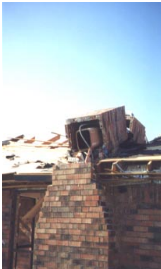
FIGURE 4-41: Close-up view brick chimney failure in Figure 4-40.
