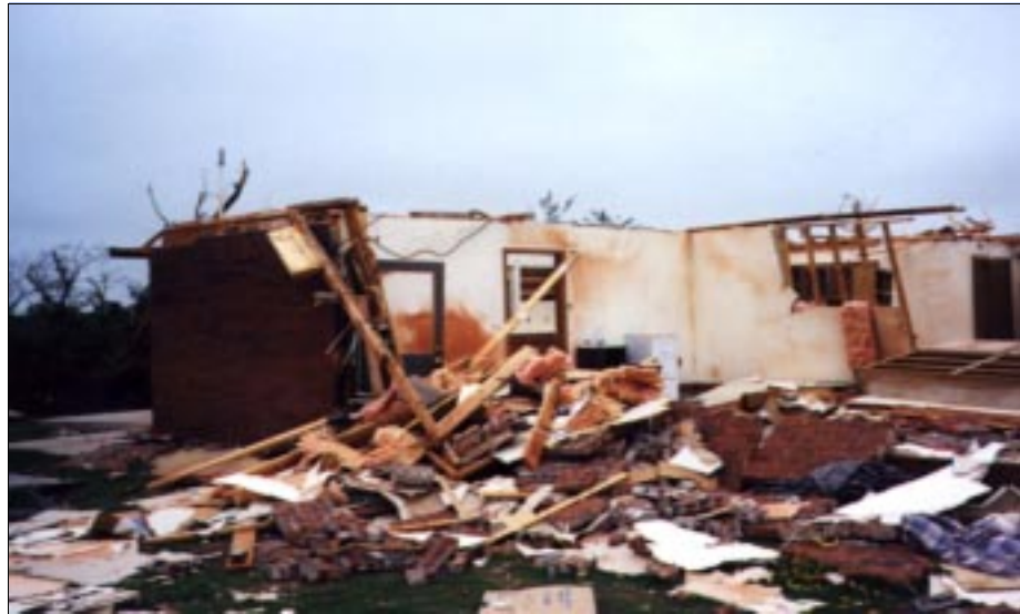
FIGURE 4-30: Failure of brick masonry veneer construction. The vortex of the severe tornado that caused the winds at this site passed approximately 30 feet from this building in Bridge Creek, Oklahoma.
