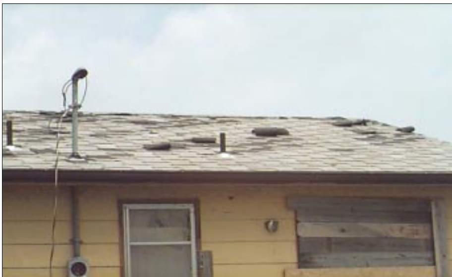
FIGURE 4-15: Several T-lock shingles on this house were lifted and torn. This house was on the periphery of the damage track left from a moderate tornado in Wichita, Kansas.
