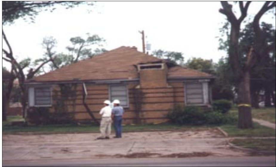
FIGURE 4-47: Chimney failure onto roof of single family attached housing located along the periphery of a severe tornado, Wichita, Kansas.
