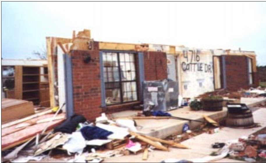
FIGURE 4-31: Brick veneer failure at the house shown in Figure 4-30.
