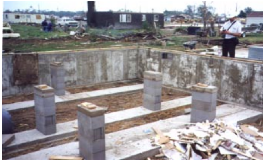
FIGURE 4-56: Lack of bolts or positive connections present between the chassis and foundation, Haysville, Kansas.
