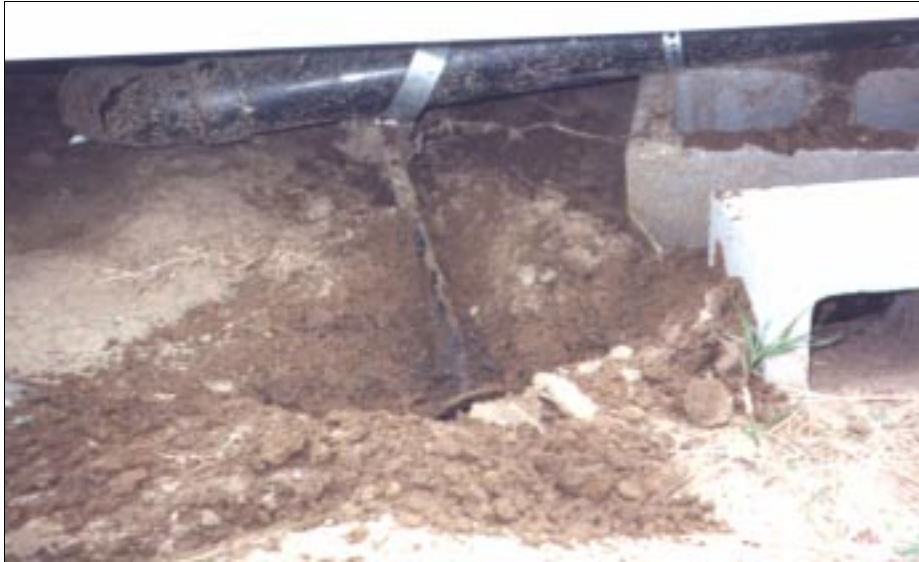
Figure 4-51: Ground anchor of manufactured home pulled from soil. This home in Wichita, Kansas, was located within the inflow area of a severe tornado.
