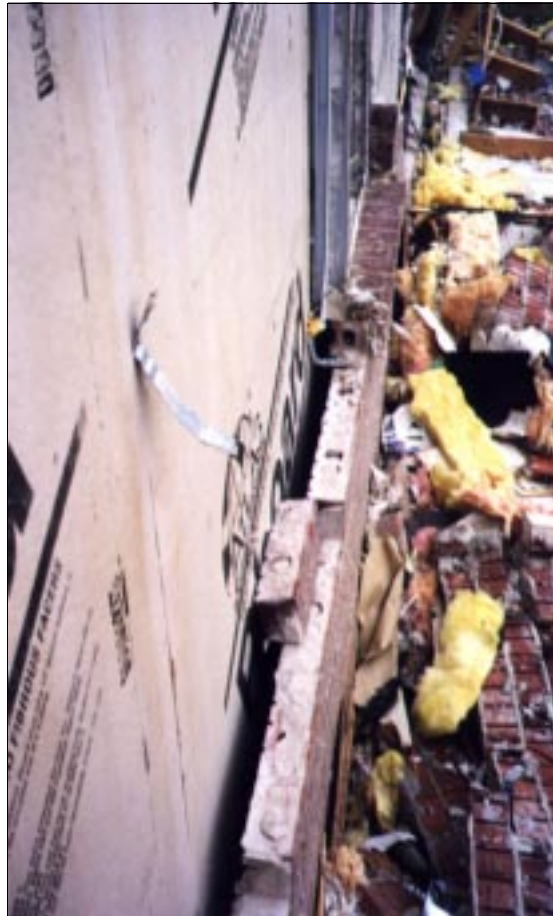
FIGURE 4-35: Inadequate bonding of mortar to galvanized brick ties, Bridge Creek, Oklahoma.
