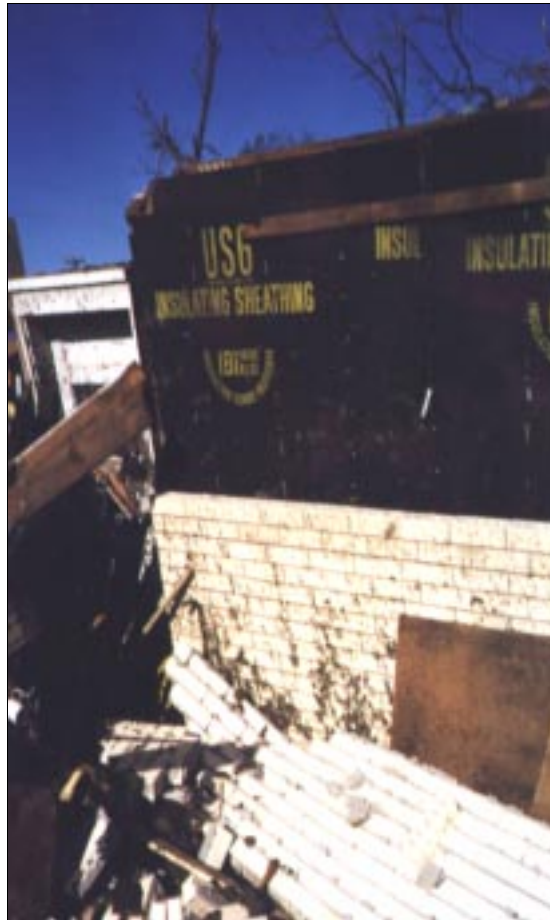
FIGURE 4-39: Failure of masonry veneer wall of home located along the periphery of a violent tornado, Del City, Oklahoma.
