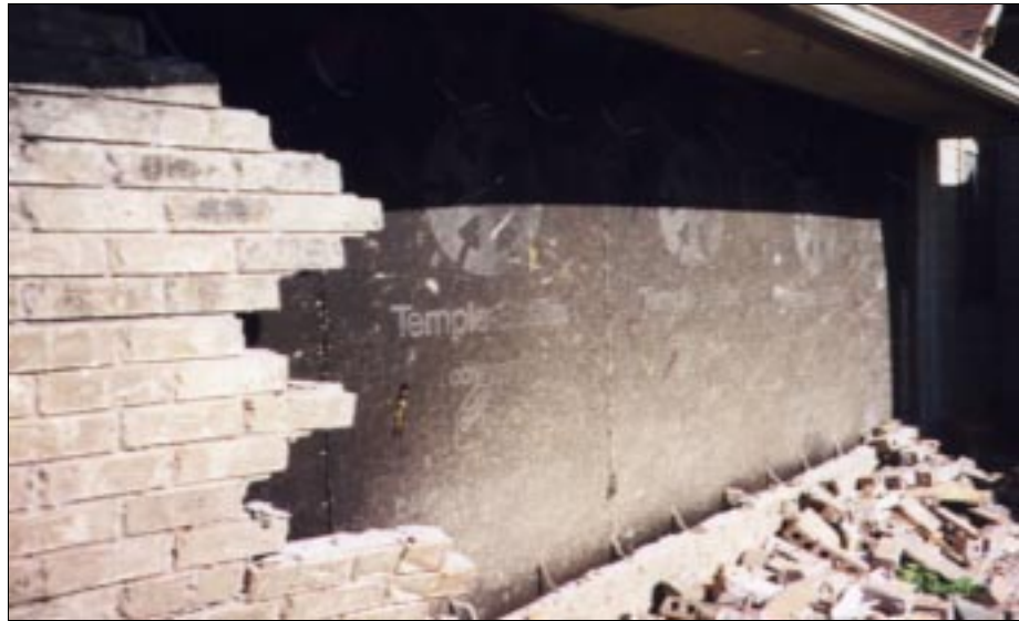
FIGURE 4-32: Failure of masonry veneer wall of a home located along the periphery of a violent tornado, Moore, Oklahoma.
