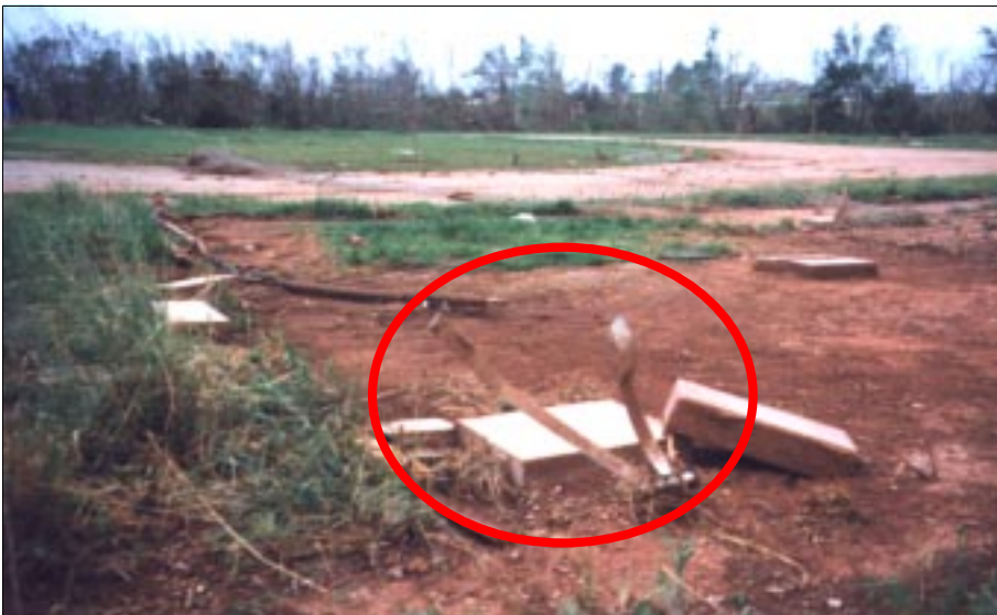
FIGURE 4-49: Failed straps at the anchorage of a manufactured home in Bridge Creek, Oklahoma. This site was 300-400 feet from a violent tornado vortex.
