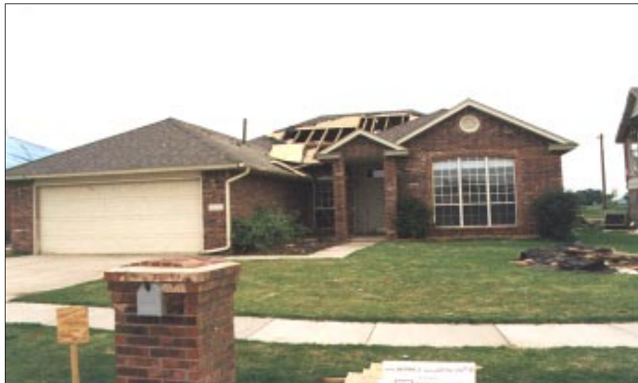
FIGURE 4-27: Front of home in Figure 4-26 where several pieces of roof decking failed.
