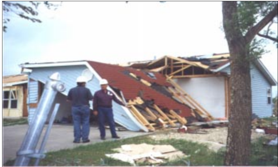
FIGURE 4-6: Wall failure due to inadequate lateral load resistance in Wichita, Kansas. The return wall at the garage inadequate to carry loads may have led to this failure.
