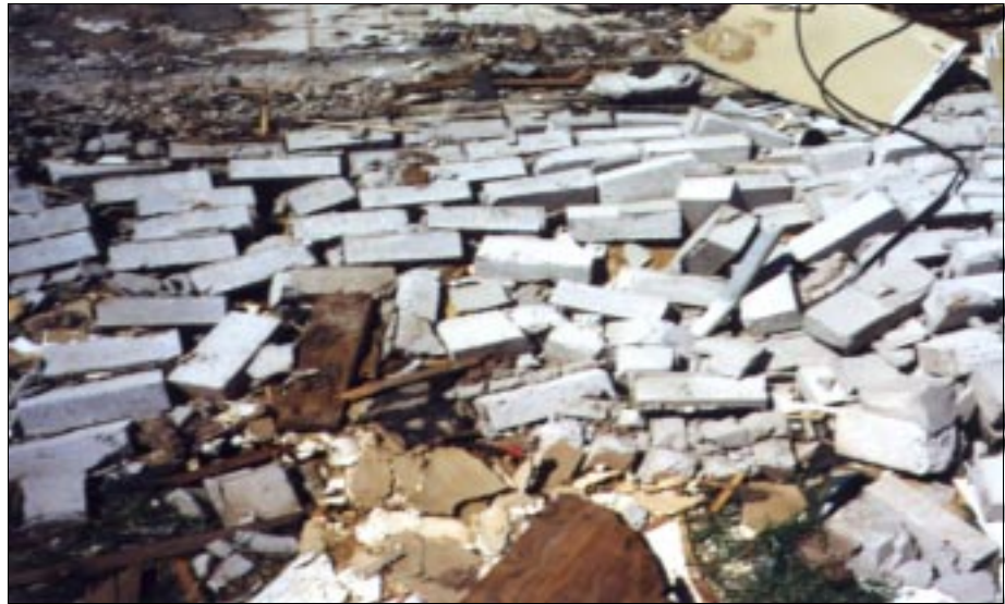
FIGURE 4-37: Failure of masonry veneer wall, viewed collapsed on the ground. This home, located in Oklahoma City was in the vortex of a violent tornado.
