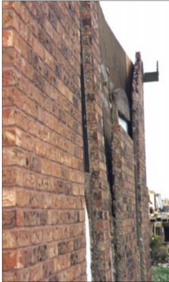
FIGURE 4-45: Failure of masonry veneer in multifamily housing located along the periphery of a severe tornado, Wichita, Kansas.
