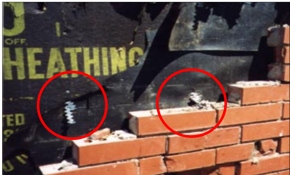
FIGURE 4-38: Failure of masonry veneer wall of home located along the periphery of a violent tornado in Oklahoma City. Masonry ties are circled.
