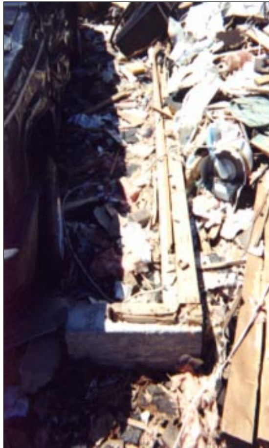
FIGURE 4-10: Wall framing to sill plate failure. This house in Del City, Oklahoma, experienced a direct hit from the vortex of a violent tornado.
