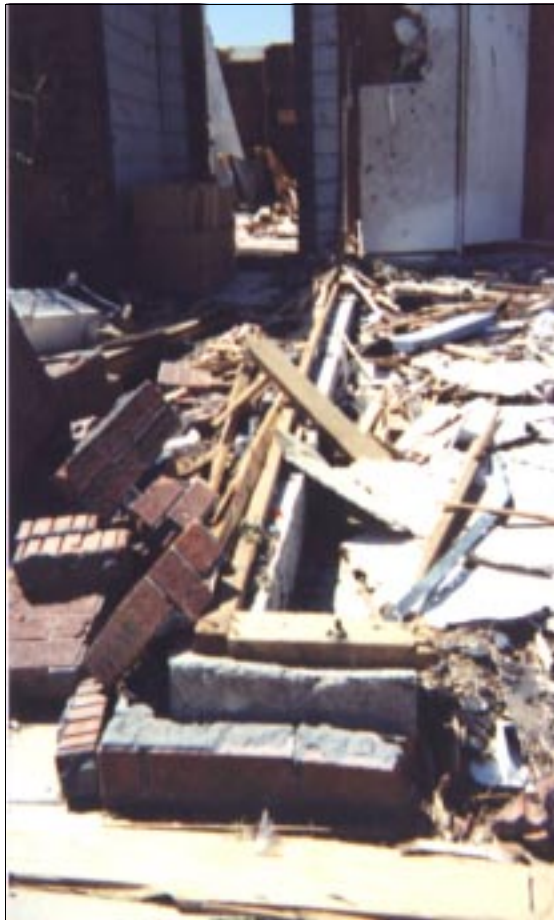
FIGURE 4-13: Failure of this sill-plate to foundation connection occurred at this home outside Oklahoma City, Oklahoma. The vortex of a violent tornado passed very close to this home.
