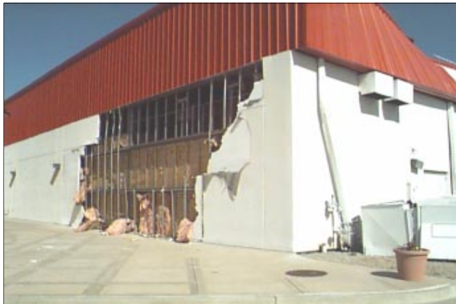
Figure 3-8: EIFS and metal component damage at the regional outlet mall in Stroud, Oklahoma.
