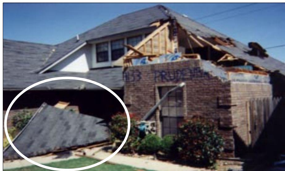
FIGURE 3-5: Failure of hip roof due to internal pressures and leeward wind forces acting together. This house, which was exposed to inflow winds of a violent tornado, was located in a suburb of Oklahoma City, Oklahoma.
