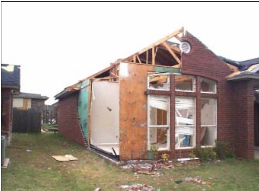
FIGURE 3-7 Failure of this exterior wall and roof section in Moore, Oklahoma, occurred when the windows broke and the front room saw an increase in internal pressure. Most of the debris from the roof and exterior wall had been cleaned up prior to this photograph. This home in Moore, Oklahoma, was located on the periphery of a violent tornado track.
