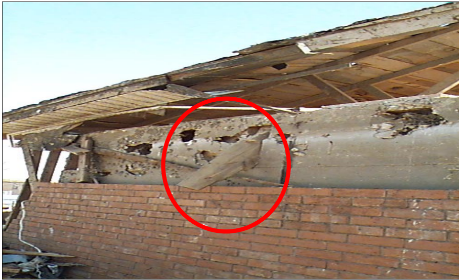
FIGURE 3-27: Several missiles struck the wall of this house in Del City, Oklahoma, including a medium sized piece of debris in the center of the picture. For scale, the square metal fastener plates near the board corners are 3-in by 3-in.
