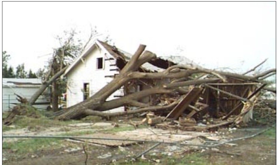
FIGURE 3-22: This building was on the periphery of a violent tornado damage area in Haysville, Kansas. One large tree fell near the corner of the house and collapsed a large portion of the roof and the corner walls. A smaller tree caused minor damage on the other corner of the house.
