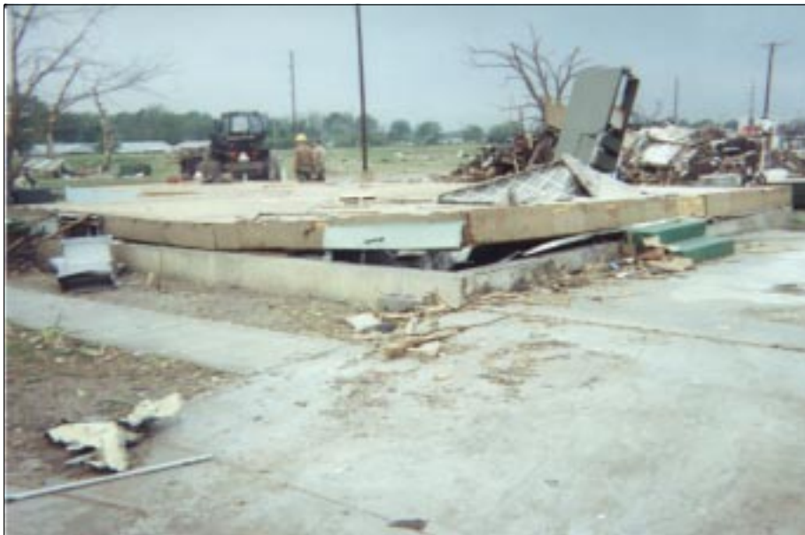
FIGURE 3-3: Wind uplift acting on this house in Haysville, Kansas, resulted in this corner of the building being lifted off its foundation.
