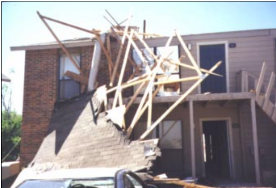
FIGURE 3-13: These trusses and roof covering (still attached to the roof sheathing) was displaced by the winds of a violent tornado and are capable of becoming large, windborne missiles.
