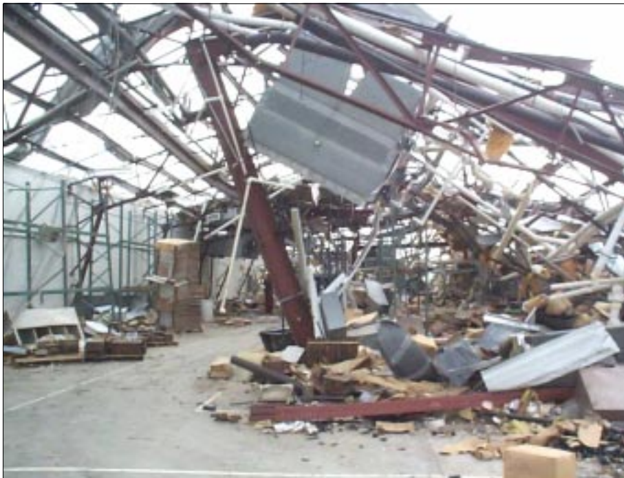
Figure 3-10: The vortex of a violent tornado passed within 100 yards of this plastics manufacturing plant in the City of Haysville, Kansas. The wind forces caused the failure of its primary structural system: a steel frame with masonry infill walls.
