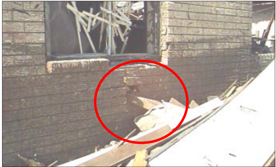
FIGURE 3-17: A 2-in by 6-in can be seen completely penetrating the brick veneer of a home in Moore, Oklahoma.
