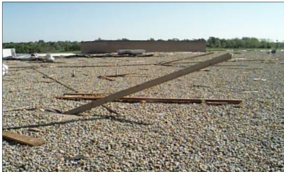
FIGURE 3-14: In the foreground, a medium sized missile, a double 2-in by 6-in, 13 feet long board can be observed sticking out of Westmoore High School's roof, Moore, Oklahoma. A larger missile, double 2-in by 10-in, 16 feet long board is lying in the background.
