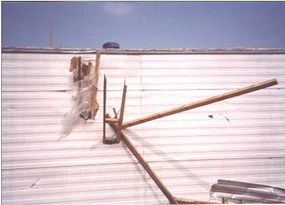
FIGURE 3-12 These medium sized missiles struck and remained embedded within this manufactured home in Wichita, Kansas.
