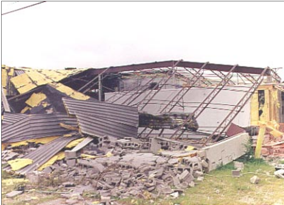
Figure 3-9: This URM wall failed when inflow winds from a severe tornado acted on this building in Wichita, Kansas.
