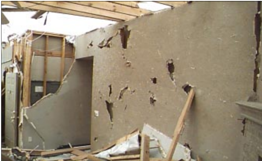
FIGURE 3-28: Several missiles struck and perforated the interior wall of this house in Moore, Oklahoma.
