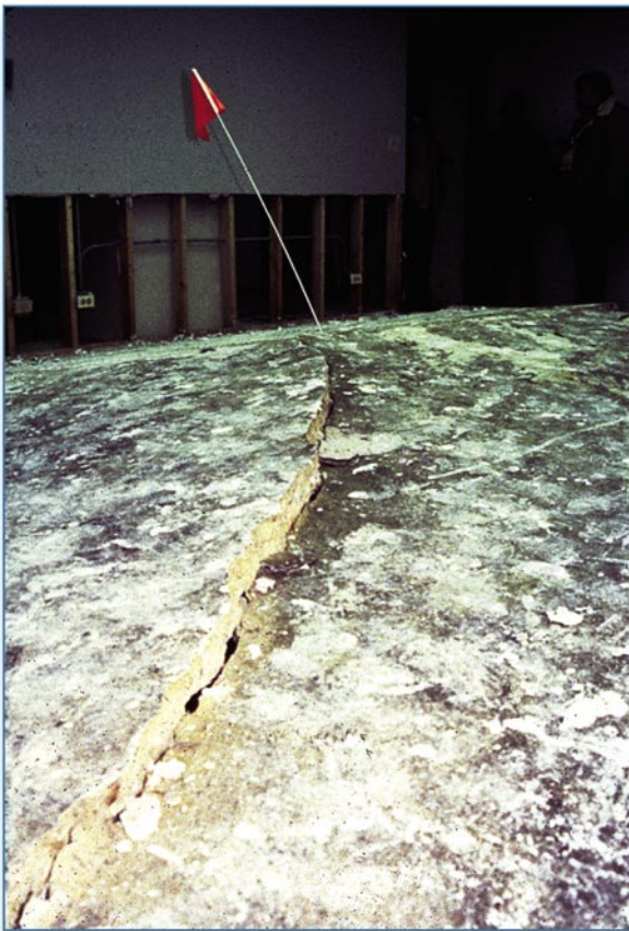
Figure 5-8 Fractured concrete basement floor, Gurnee, IL, 1986
