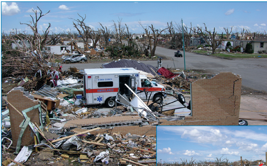
Figure 4-141: View of the collapsed ambulance garage. The twin-tees (red arrows) flew to the left, as shown in the inset.
