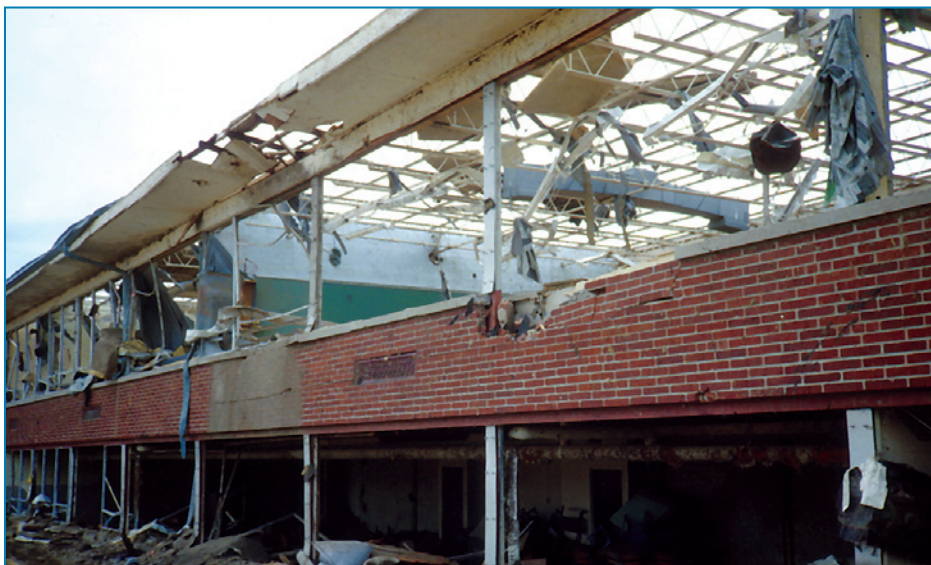
Figure 4-12: This building in Northern Illinois was heavily damaged by a strong tornado in 1990.
