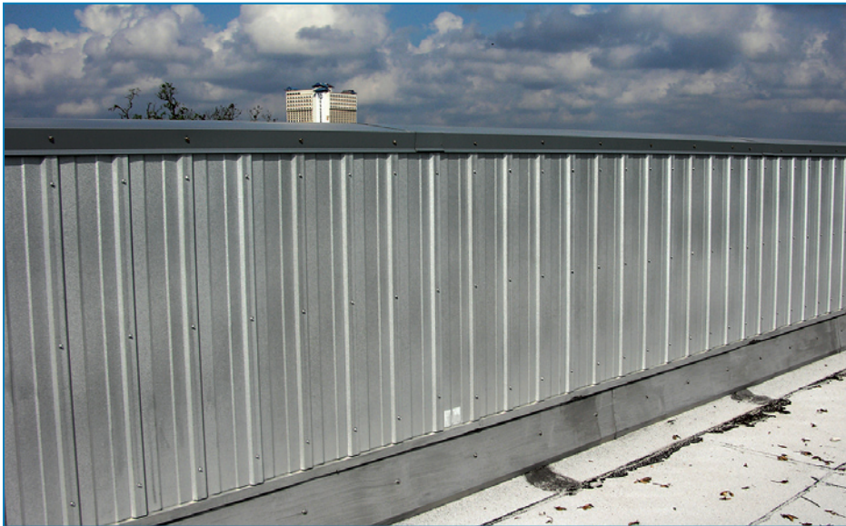
Figure 4-79: Base flashing protected by metal panels attached with exposed screws. Hurricane Katrina (Mississippi, 2005)
