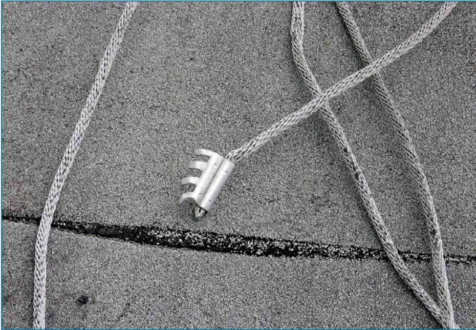
Figure 4-104: If conductors detach from the roof, they are likely to pull out from pronged splice connectors. Hurricane Charley (Florida, 2004)
