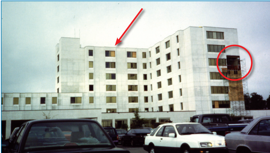
Figure 4-11: Collapse of non-load-bearing wall (red circle) and broken glazing from roof aggregate (red arrow). Hurricane Hugo (South Carolina, 1989)
