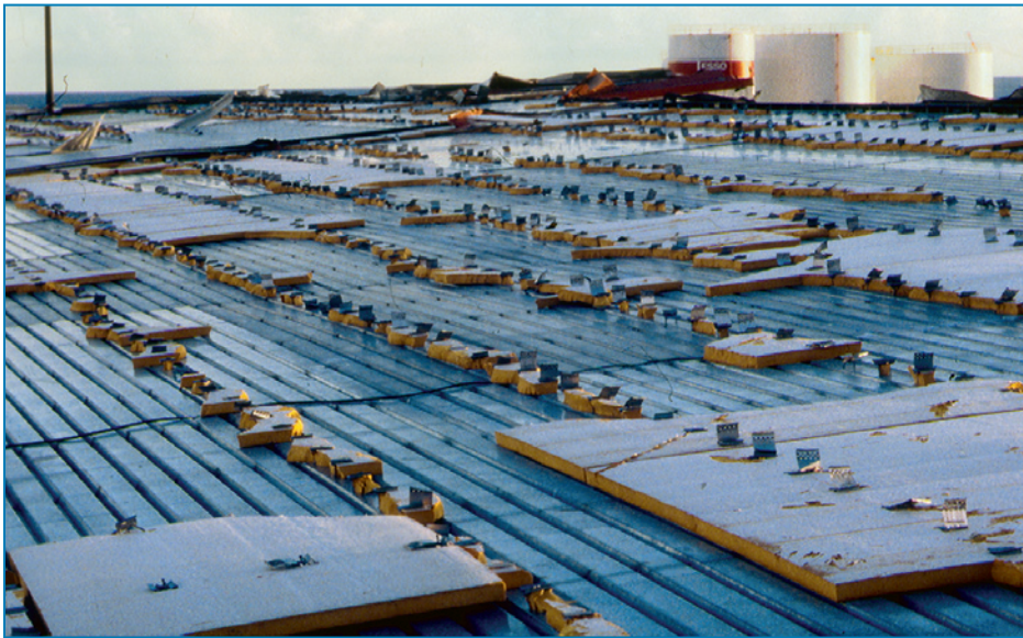
Figure 4-73: Significant interior water damage and facility interruption occurred after the standing seam roof blew off. Hurricane Marilyn (U.S. Virgin Islands, 1995)
