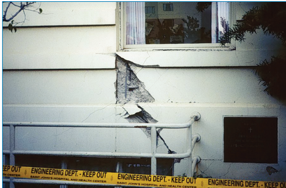
Figure 2-19: Damage to an exterior concrete wall. This hospital building was evacuated.
