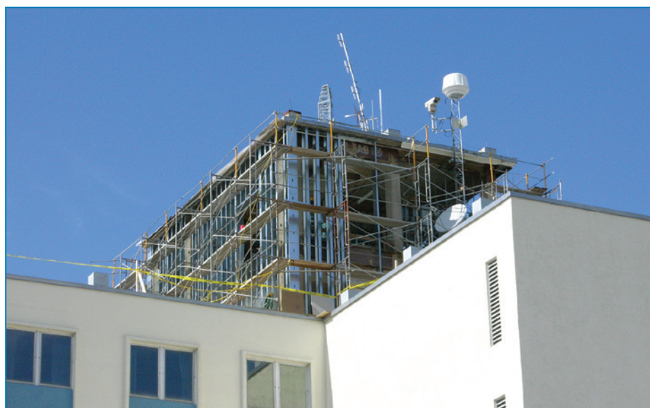
Figure 4-106: View of the reconstruction of the damaged walls at the elevator penthouse
