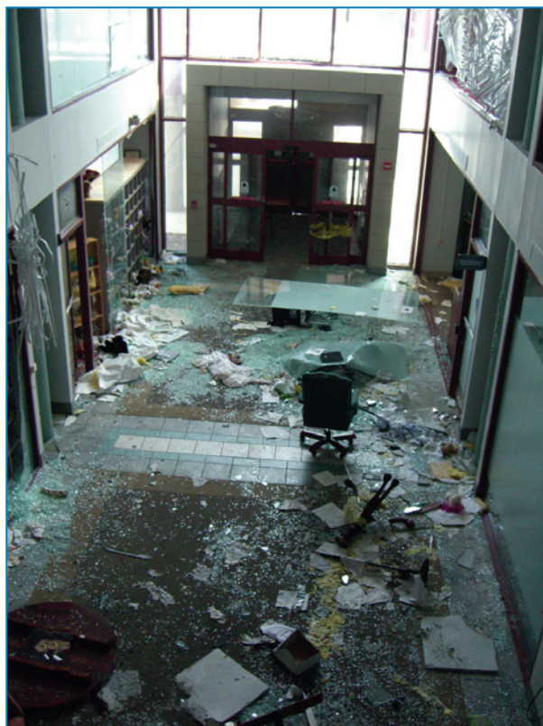
Figure 4-147: Glass shards and other debris in the lobby area housing retail shops and offices.
