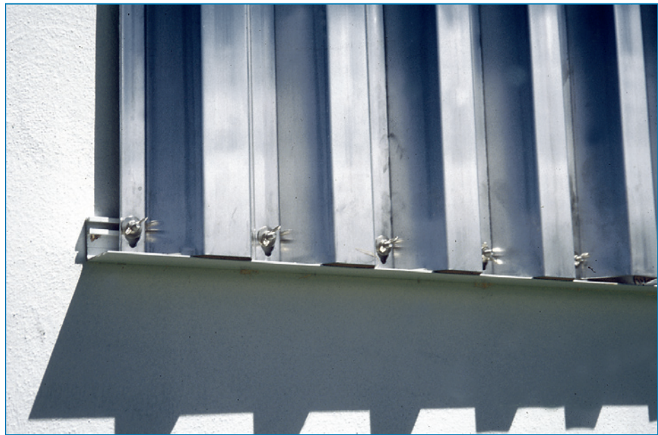
Figure 4-117: A metal panel shutter. Hurricane Georges (Puerto Rico, 1998)
