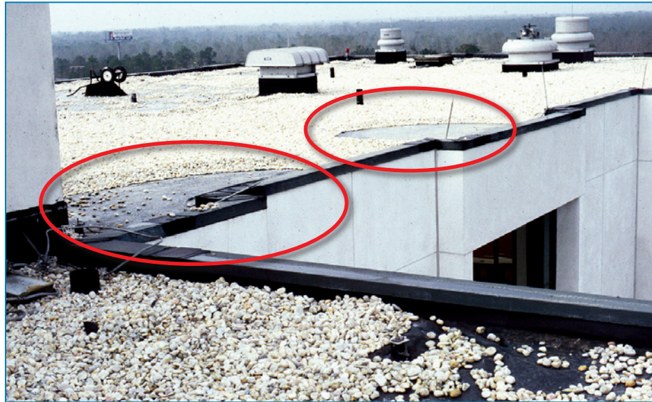
Figure 4-5: Aggregate blow-off associated with building irregularities. Hurricane Hugo (South Carolina, 1989)
