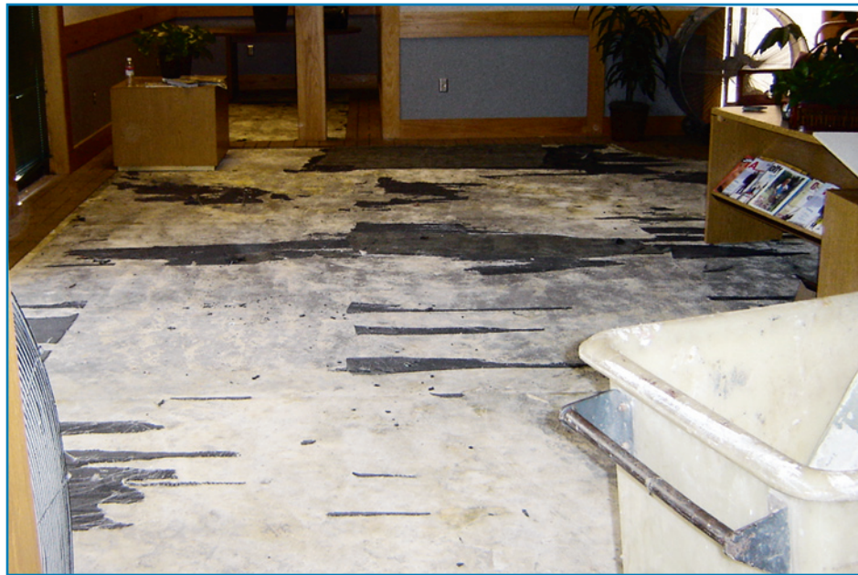
Figure 3-19: Floor damage at West Jefferson Medical Center (Hurricane Katrina, 2005)
