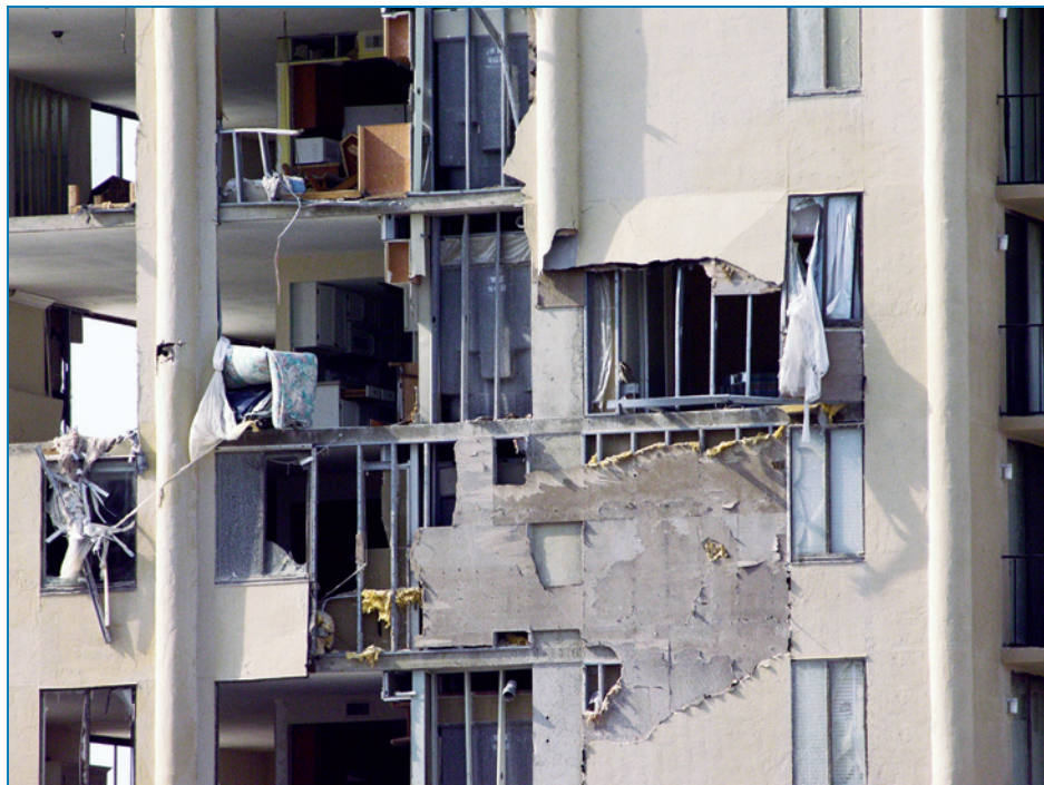
Figure 4-61: The stucco wall failure was caused by inadequate attachment between the stud tracks and the building's structure. Hurricane Ivan (Florida, 2004)
