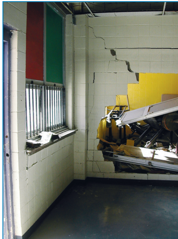
Figure 3-14: Interior unreinforced masonry walls of the Port Sulphur High School in Louisiana were damaged by hydrostatic loads associated with Hurricane Katrina's storm surge (2005).
