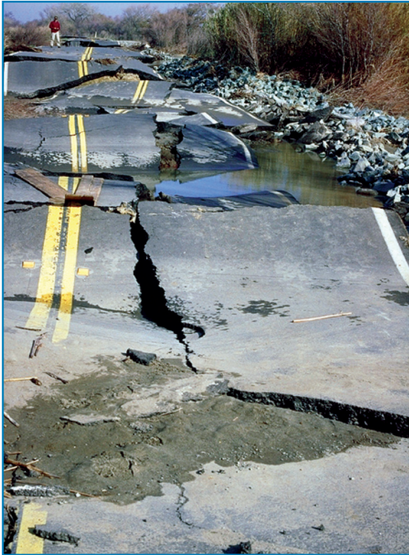
Figure 3-13: Flooding caused the failure of this road bed.
