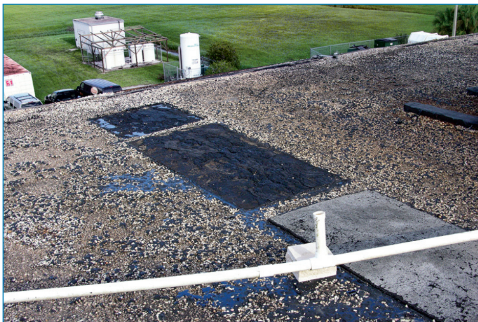
Figure 4-82: View of the back side of the third floor roof where the gutter and an asphalt plank walkway pad were blown away. The loose aggregate surfacing was also blown away.
