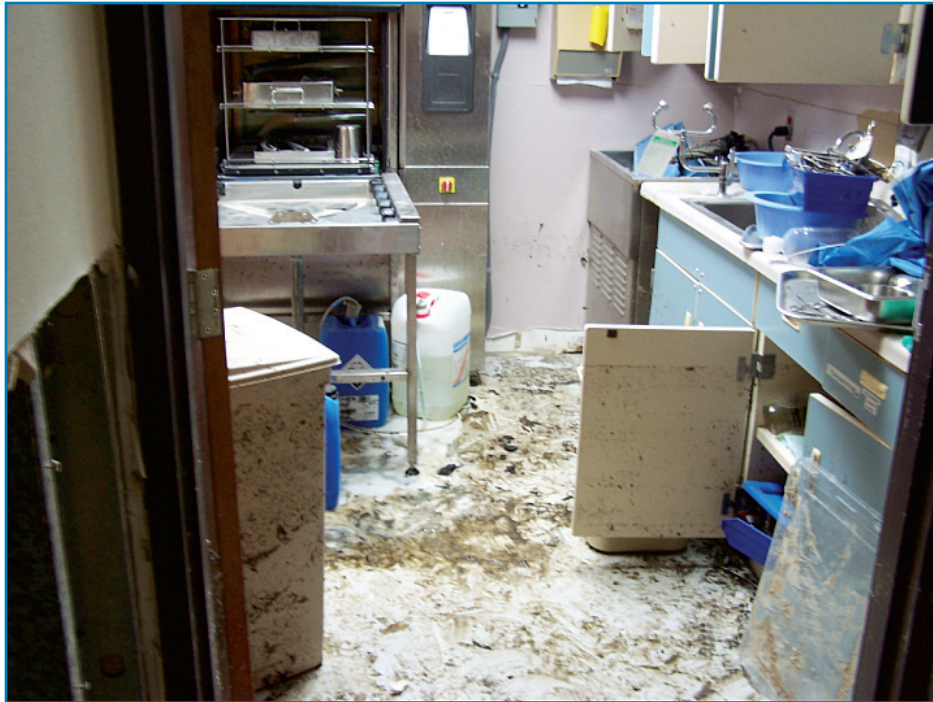
Figure 3-23: The interior of the Hancock Medical Center required extensive cleanup following flooding (Hurricane Katrina, 2005).
