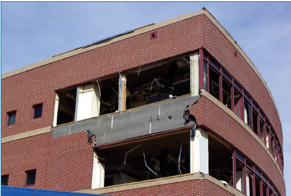
Figure 4-146: Several of the window frames were blown away, along with some of the brick veneer (1999 addition).
