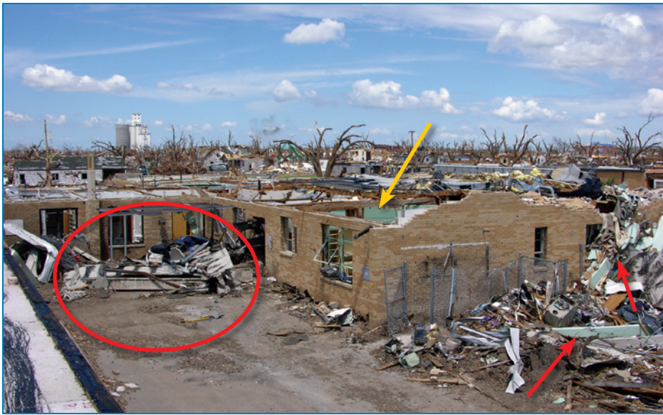
Figure 4-133: The missing tee shown in Figure 4-132 landed about 80 feet away (red oval). The red arrows show tees that were blown from the ambulance garage. Note the missing wood roof structure on the 1982 addition (yellow arrow).
