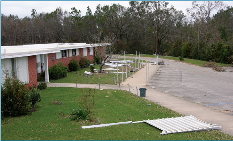
Figure 4-33: The destroyed walkway canopy in front of this building became wind-borne debris. Hurricane Ivan (Florida, 2004)
