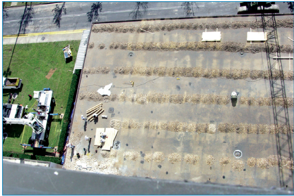
Figure 4-20: Looking down at the one-story roof to the right of the MOB in Figure 4-19. The small dark areas are locations where emergency patches had been placed to repair punctures from falling glass shards. (Note: At the time the photo was taken, the ballast had been repositioned into rows in preparation for removal)
