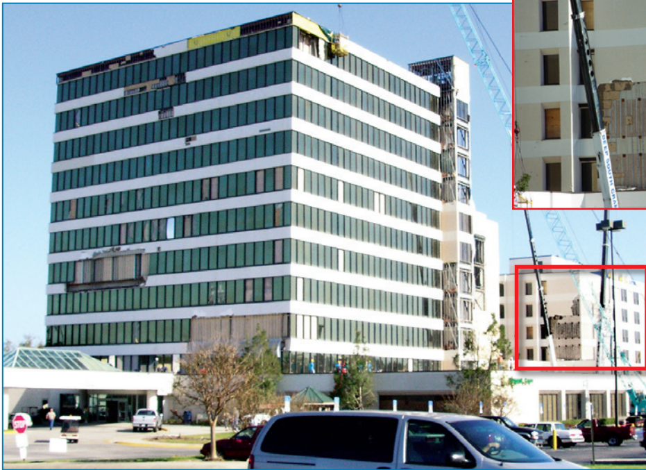
Figure 4-19: EIFS debris blown off the hospital building (Item J on Figure 4-13) in the background (red square) broke numerous windows in the MOB (item G on figure 4-13) in the foreground.
