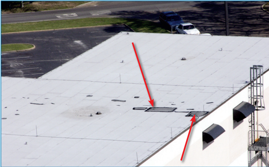
Figure 4-14: Numerous repairs where the modified bitumen roof membrane was punctured by missiles. Water from the punctured membrane entered the surgical suite.
