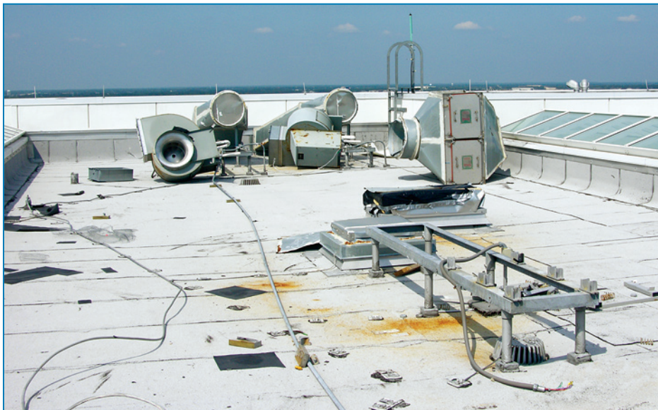
Figure 4-25: Temporary coverings placed over two large openings in the roof that were left after the ductwork blew away. Hurricane Katrina (Mississippi, 2005)
