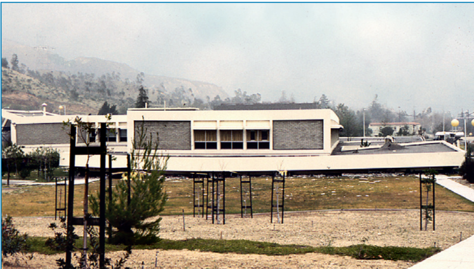
Figure 2-22: Completely collapsed first level (not visible) of Psychiatric Unit
