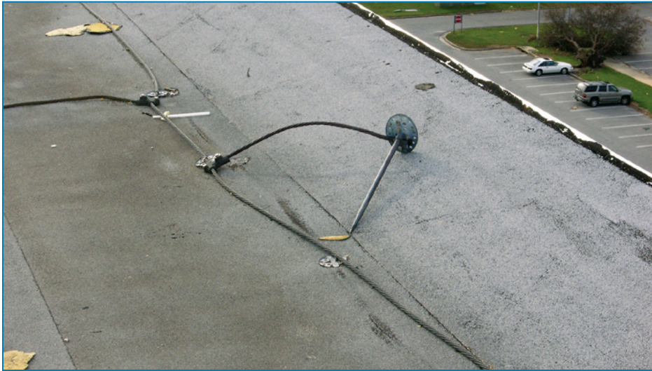
Figure 4-98: An air terminal debonded from the hospital's roof. Displaced air terminals can puncture tough membranes, such as this modified bitumen membrane. Hurricane Ivan (Florida, 2004)
