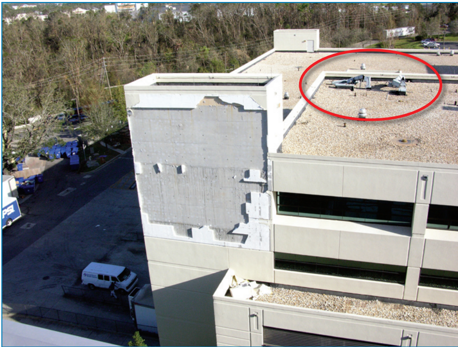
Figure 4-60: EIFS blown off a cast-in-place concrete wall. Note the damaged rooftop ductwork. Hurricane Ivan (Florida, 2004)
