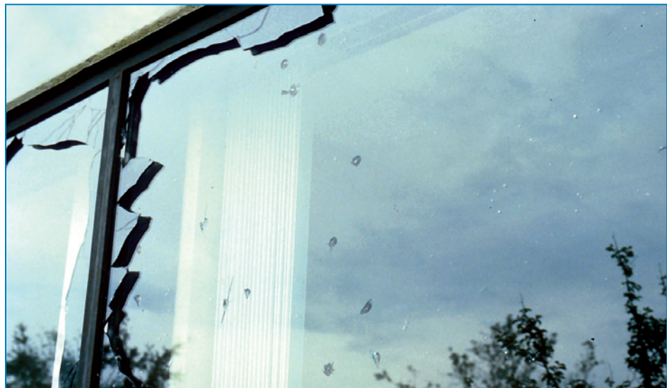
Figure 4-10: The outer window panes were broken by aggregate from a built-up roof. Hurricane Hugo (South Carolina, 1989)
