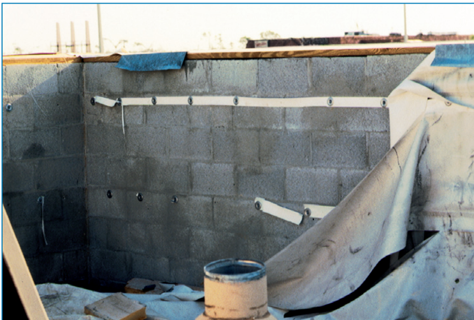
Figure 4-70: If mechanically attached base flashings have an insufficient number of fasteners, the base flashing can be blown away. Hurricane Andrew (Florida, 1992)
