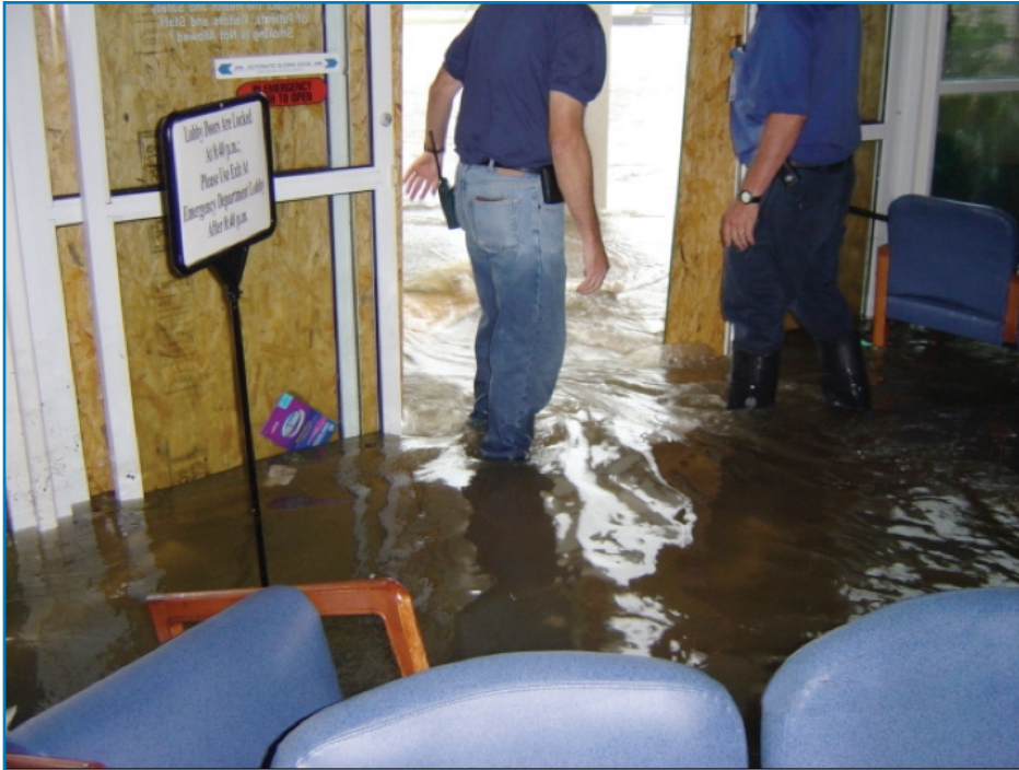
Figure 3-49: Flooding at Hancock Medical Center during Hurricane Katrina
