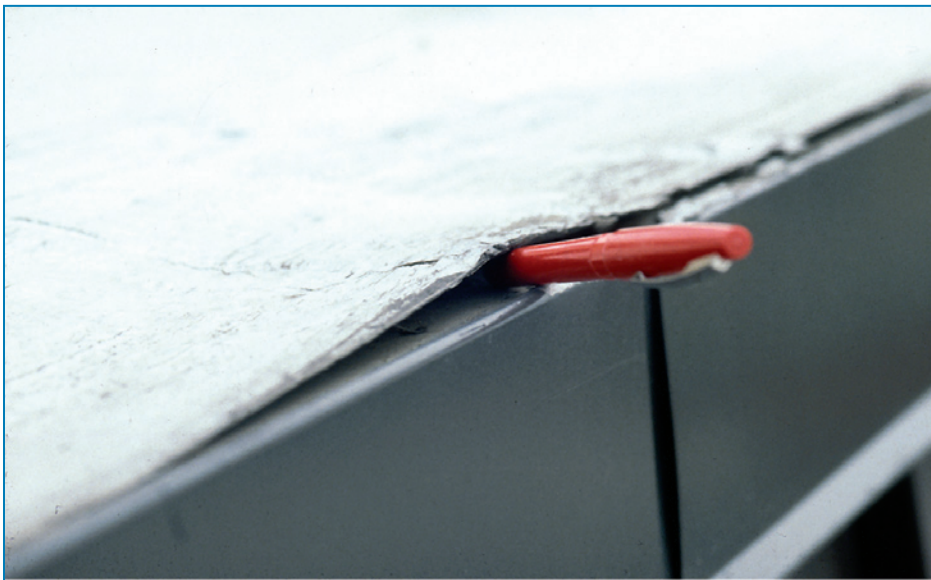
Figure 4-65: The ink pen shows an opening that the wind can catch, and cause lifting and peeling of the membrane.
