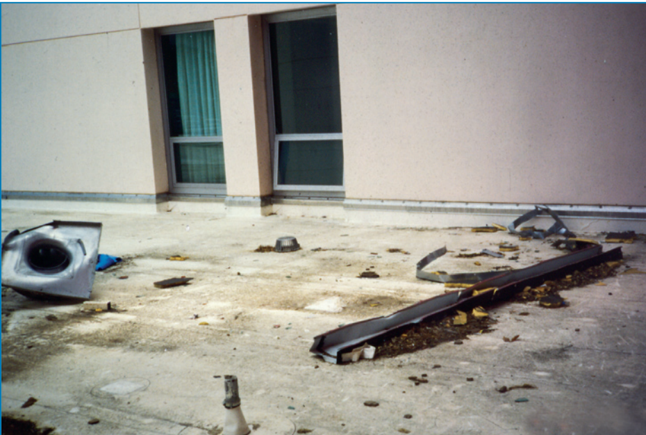
Figure 4-76: This fully adhered single-ply roof membrane was struck by a variety of missiles. Hurricane Marilyn (U.S. Virgin Islands, 1995)
