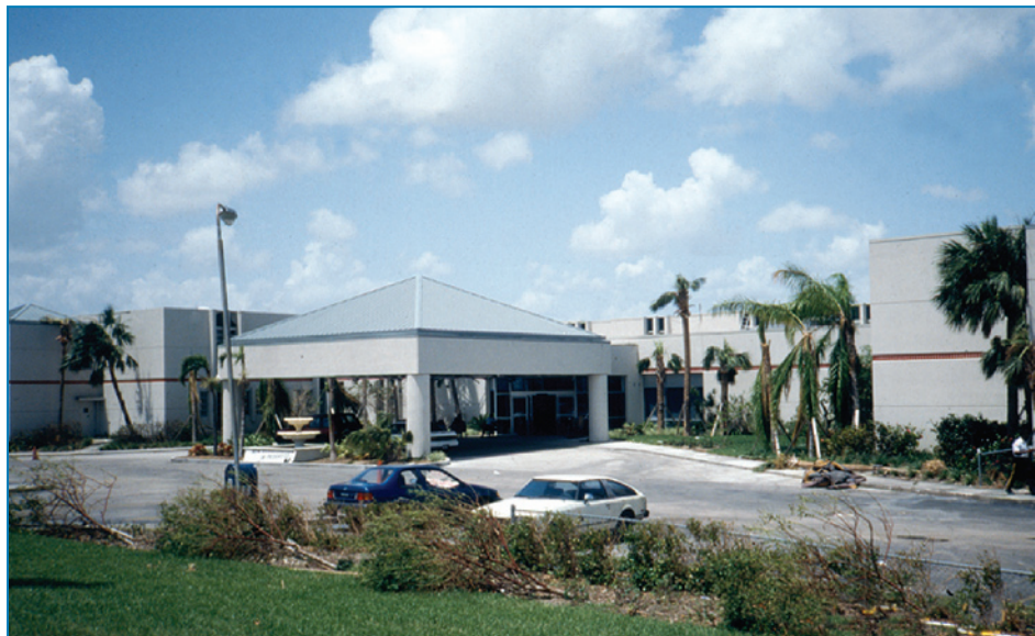
Figure 4-1: Deering Hospital was evacuated after Hurricane Andrew due to water infiltration caused by roof covering, window, and door damage.
