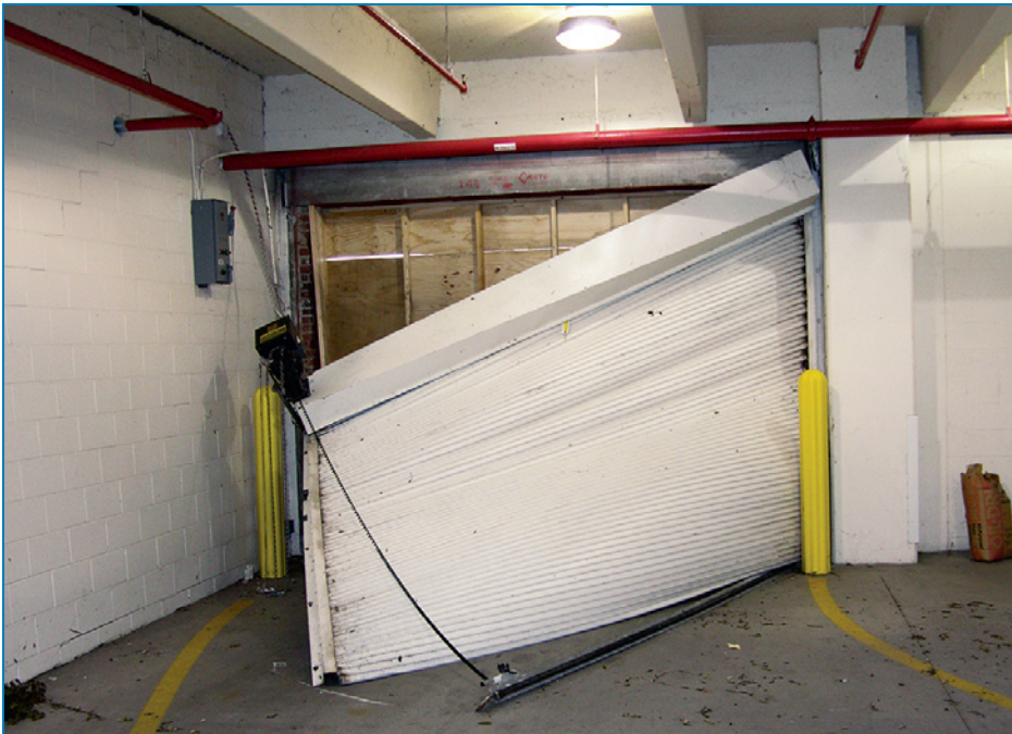
Figure 4-35: This new rolling door failed because the CMU spalled at the door frame's expansion bolts, which were too close to the end of the CMU. Hurricane Charley (Florida, 2004)
