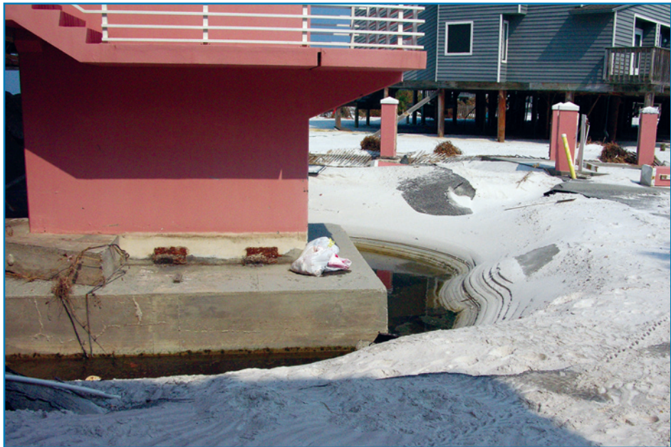
Figure 3-17: Local scour undermined the footing of this exterior stair tower (Hurricane Ivan, 2004).
