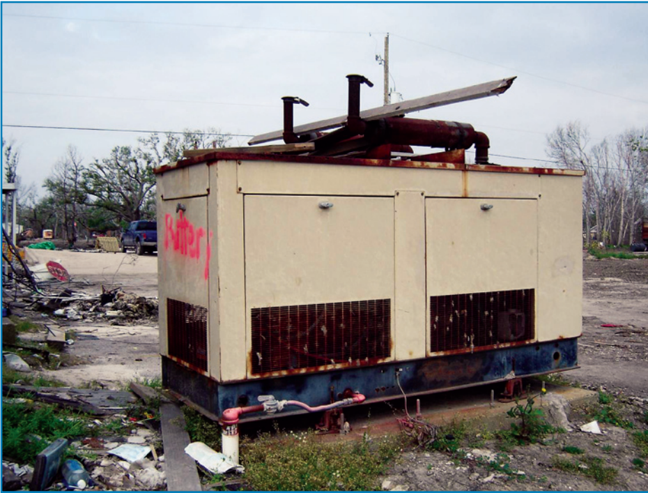
Figure 3-21: Although it was anchored and not displaced by floodwaters, this generator was out of service after being submerged (Hurricane Katrina, 2005).
