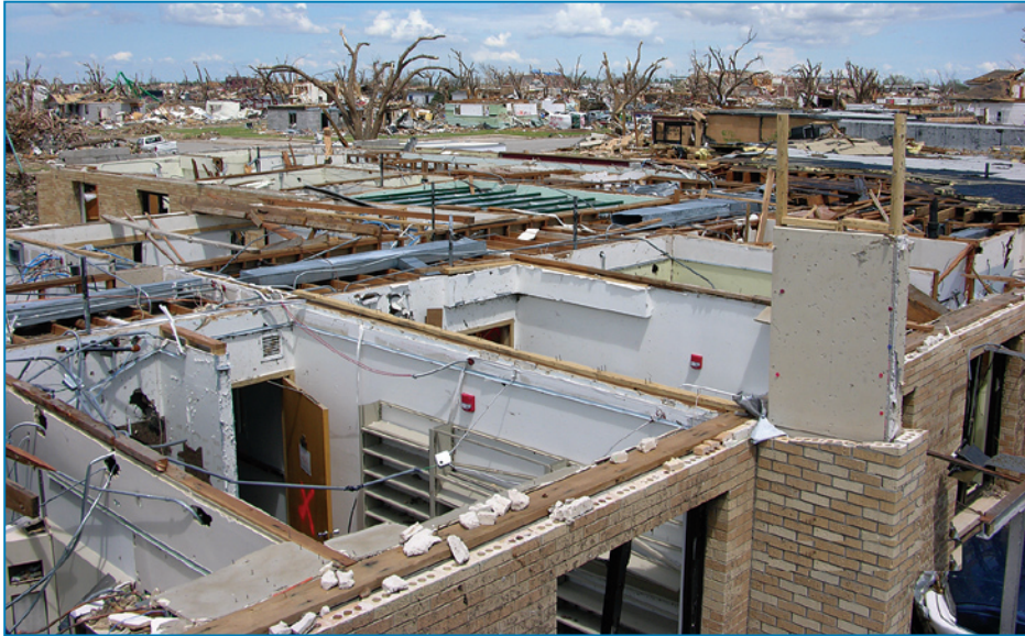
Figure 4-140: Loss of the wood roof structure at the 1982 addition.
