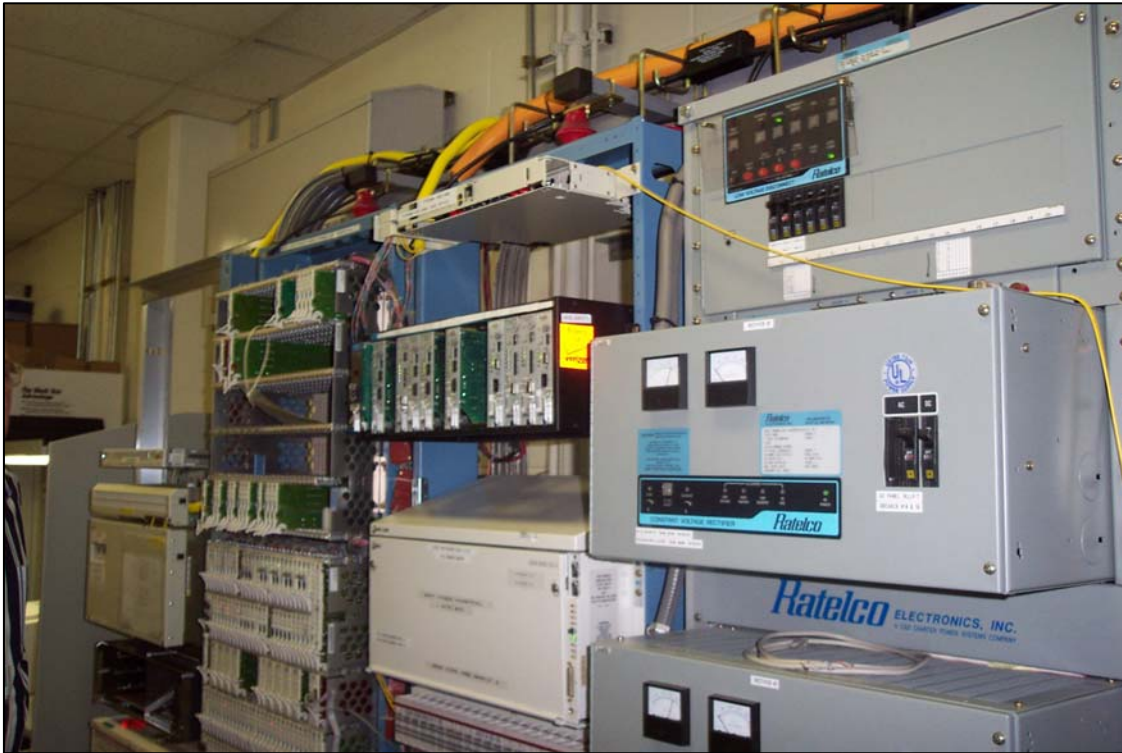
Figure 25. Telecom and Network Equipment
