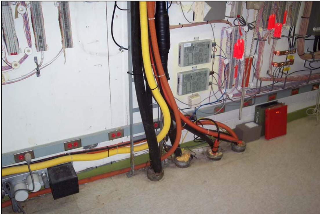
Figure 24. Telecom and Network Cabling
