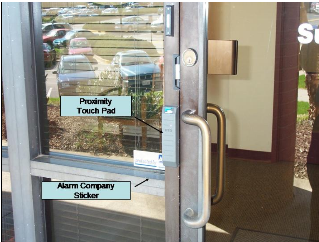
Figure 27. Proximity Card Reader and Alarm Sticker
