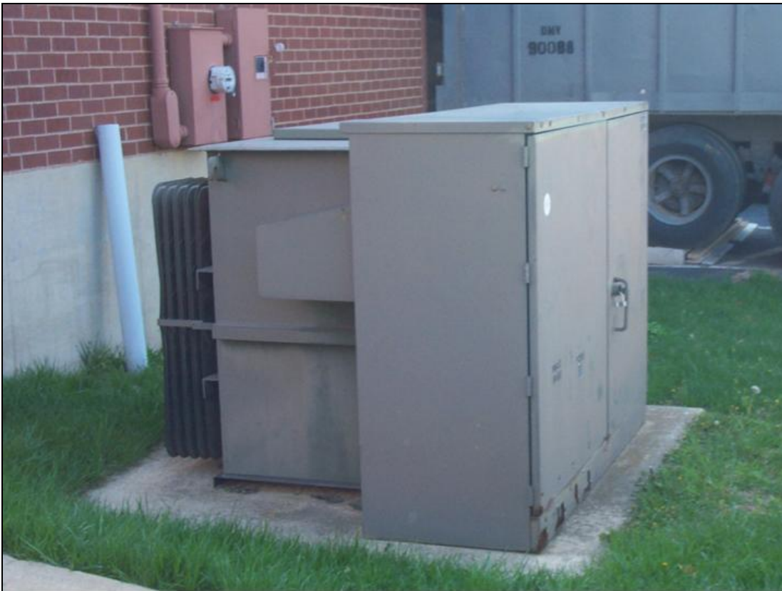
Figure 20. One of Two Transformers On Site
