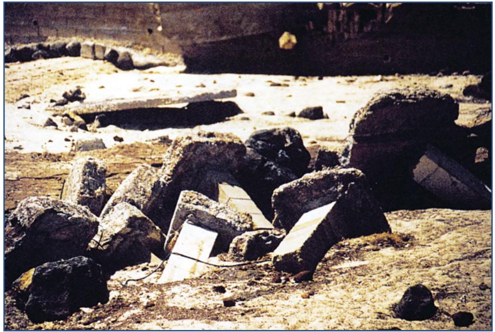
The small footings on the piers in this photograph did not prevent these piers from overturning during Hurricane Iniki.
