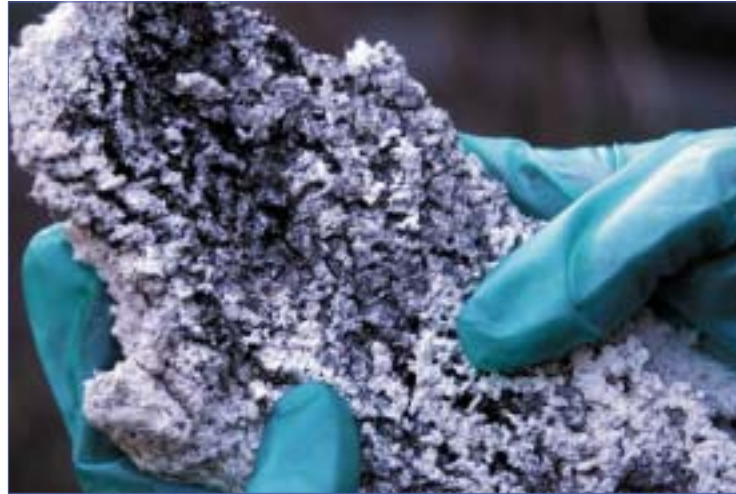
Mold, like that growing on a piece of ceiling tile shown above, can gradually destroy the things they grow on. The EPA's fungal detection technology can help prevent further damage to homes, save money, and avoid potential health problems.
