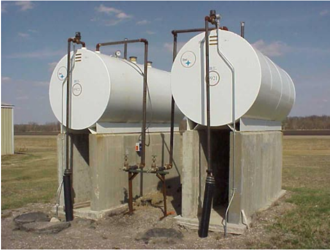
New 2,000-gallon aircraft fuel tanks now are elevated and secured to concrete bases to ensure they don't float away in another flood.
