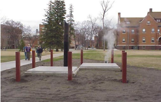
University of North Dakota steam lines now are better protected from future flood damage.
