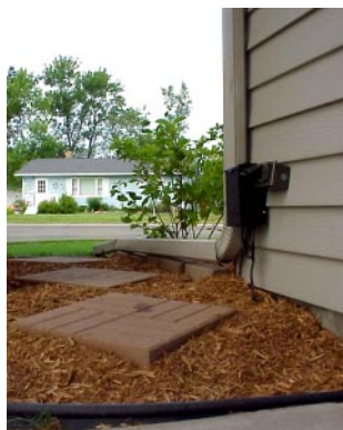
More pavers outside Styf's garage also help direct water away from the structure and foundation.
