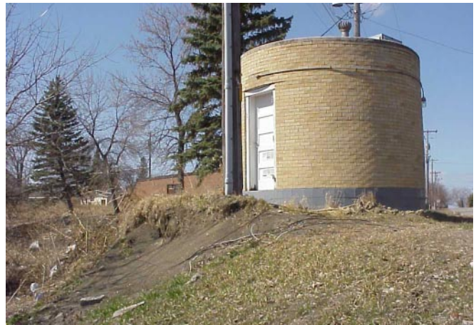
The old master lift station sits dangerously close to the edge of the riverbank.
