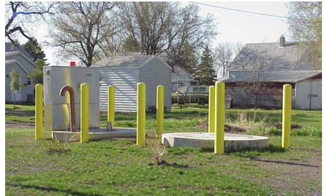
A new master lift station has been built away from the river in an area that now can be better protected from flooding. Removing the old lift station from the edge of the riverbank also enables the city to construct temporary dikes to keep floodwaters getting into town.
