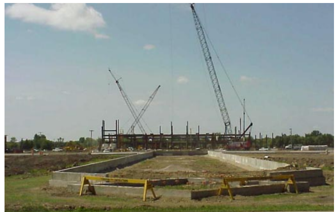
The new Engelstad Arena will better weather future storms because of several added disaster-resistant features.
