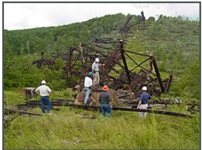
FEMA personnel examine the Kinzua Bridge in Lackawanna County, Pa., after a tornado destroyed it on July 21.
