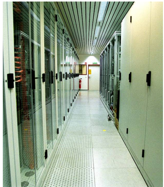
Network Equipment Room at the Columbus Control Center
