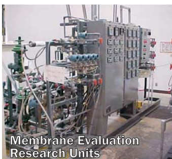
Portable Chemical Feed Systems
