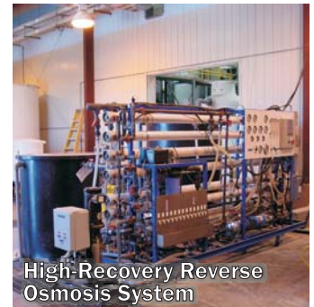
Pilot-scale membrane pretreatment system
