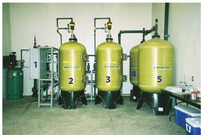
Figure 2. Macrolite® Pressure Filtration System (Control Panel [1], Macrolite® Filters [2, 3], and Contact Tanks [4, 5])
