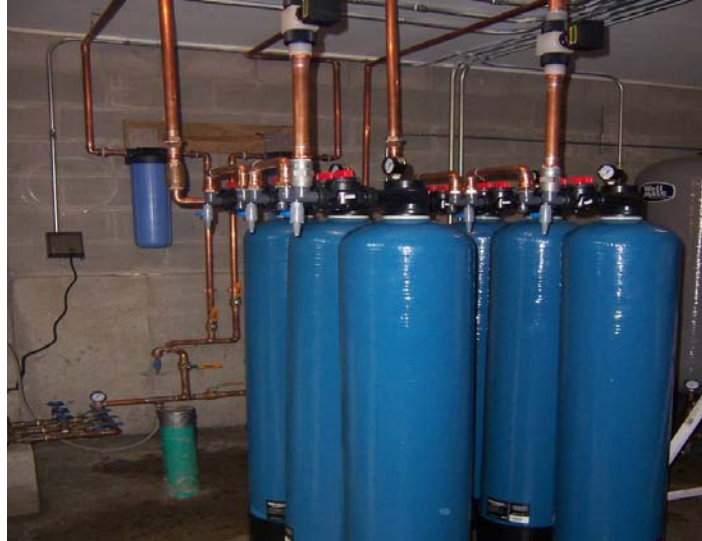
Figure 4-5. As/2200CS System with Adsorption Columns Shown in Foreground and Sediment Filters Attached to Wall
