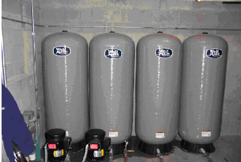
Figure 4-2. Preexisting Pressure Tanks and Booster Pumps
