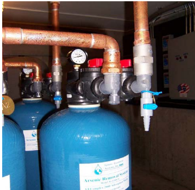
Figure 4-6. Close-Up View of a Sample Tap (TE), a Pressure Gauge, and Copper Piping at End of Treatment Train A
