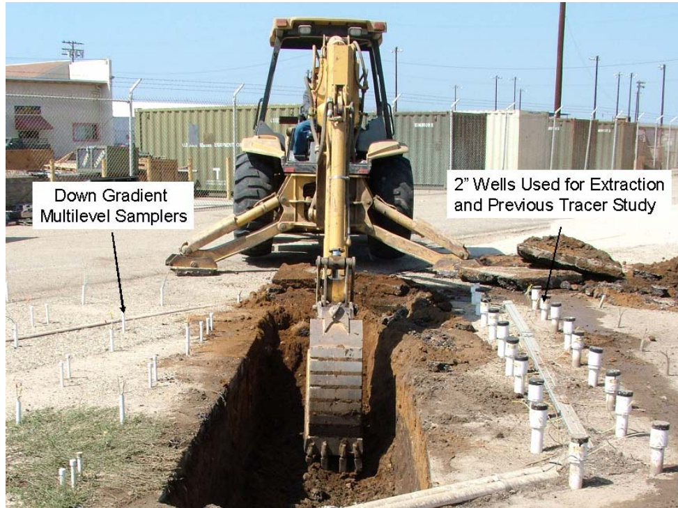
Figure 5. Removal of 1.2 m of the existing formation material to allow for the construction of the infiltration gallery.
