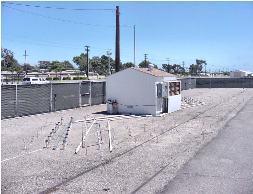
Figure 4. Location of north infiltration gallery showing Envirogen gas injection wells prior to the beginning of work.
