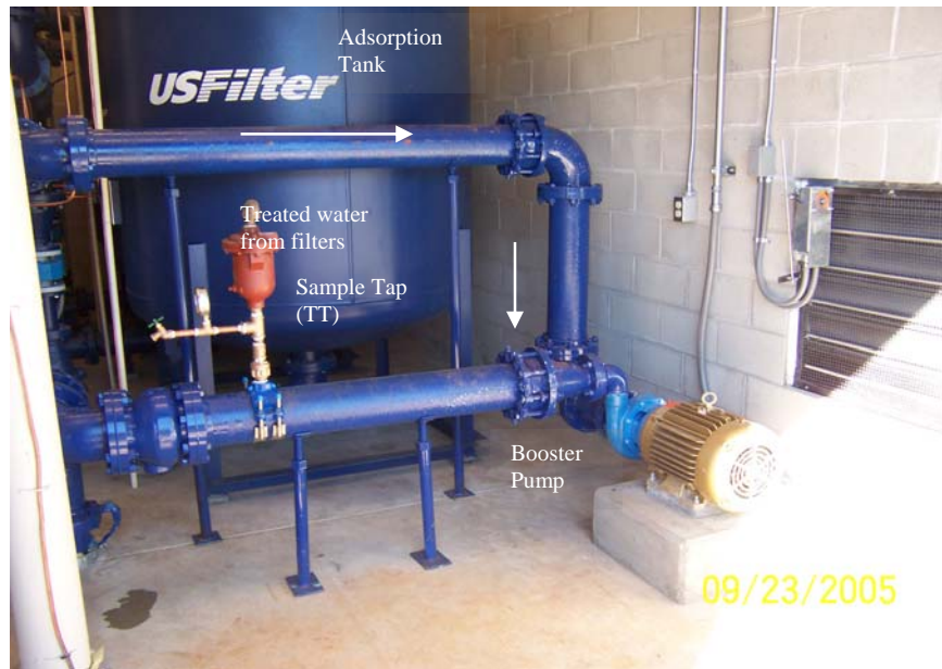
Figure 4-5. A New Booster Pump Station
