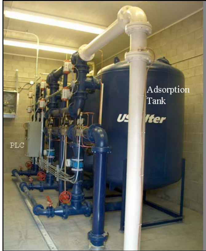
Figure 4-4. Siemens GFH Arsenic/Antimony Removal System
