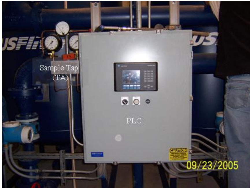
Figure 4-7. Programmable Logic Controller
