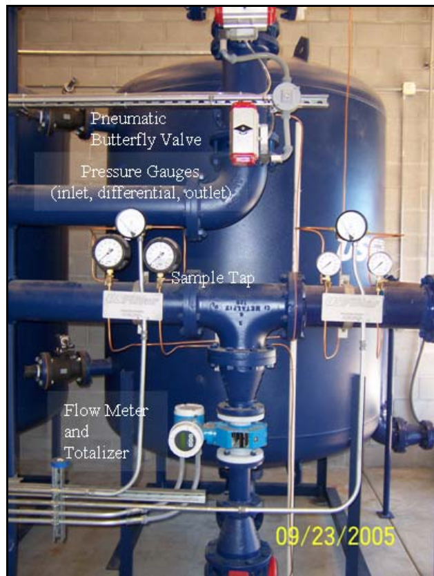
Figure 4-8. Third Pressure Vessel and Associated Plumbing and Monitoring Components
