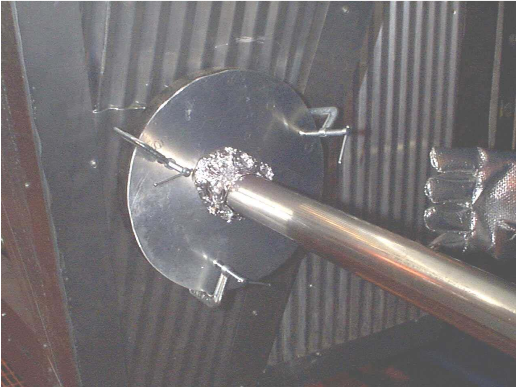
Figure 4-2. Dilution system sampling probe installed in 6 in. I.D. flanged port.
