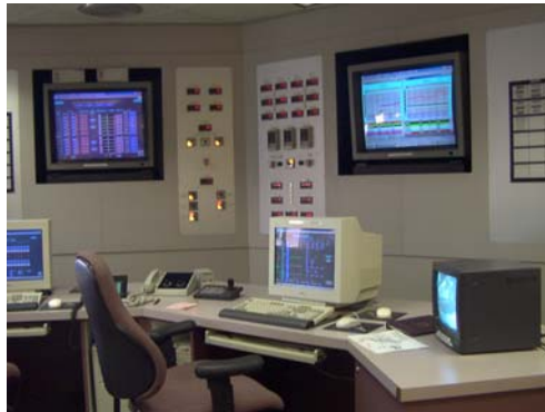
Figure 5-1. Picture of a SCADA control console.
