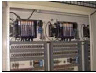
Figure 5-4. Picture of a typical PLC.
