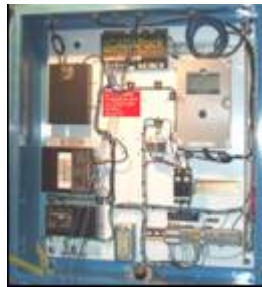
Figure 5-5. Picture of a typical RTU panel.
