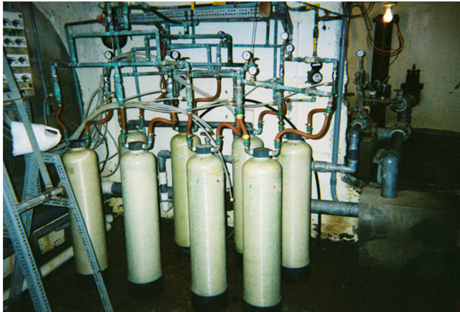
Figure 4-3. Existing Activated Alumina System in the Underground Treatment and Control Structure
