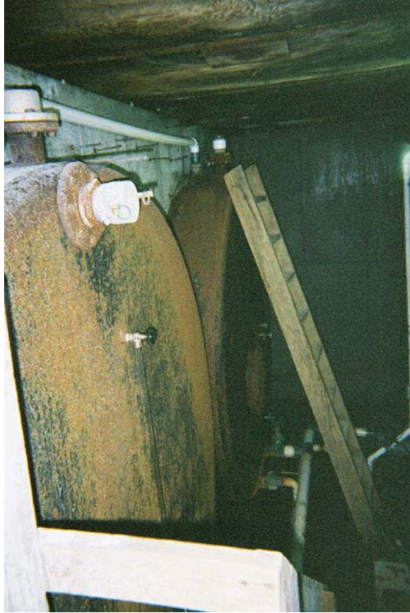
Figure 4-2. Existing Storage Tanks in Underground Concrete Structure
