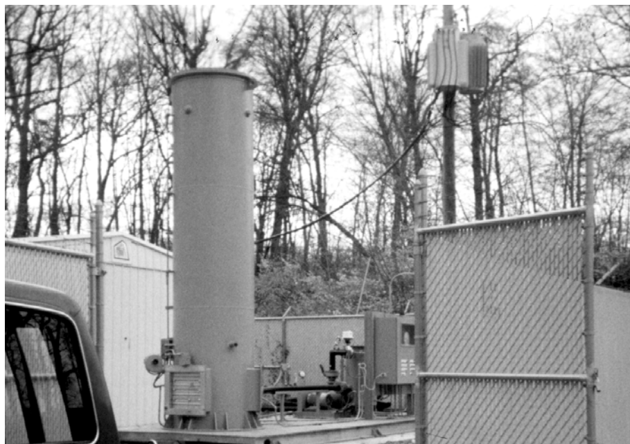
Figure 5-8. Small Skid-Mounted Enclosed Ground Flare.
