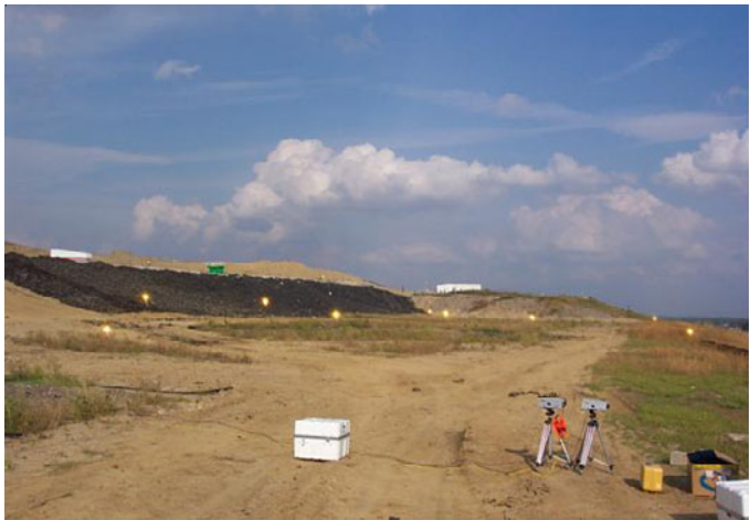
Figure 6. HRPM Configuration Used to Survey the As-Built Lower Cell During the May 2003 Field Campaign.
