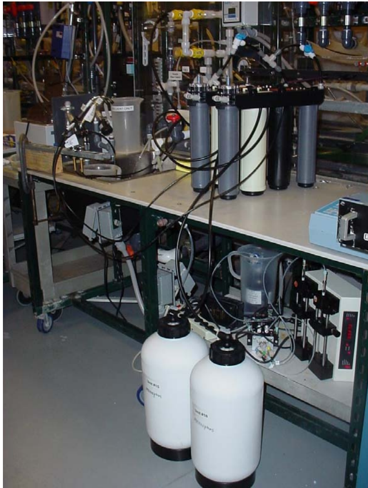
Figure 3-1. RO Membrane Systems Installed at a Test Station
