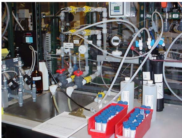
Figure 3-2. Post-Membrane Carbon Filters Installed at a Test Station.
