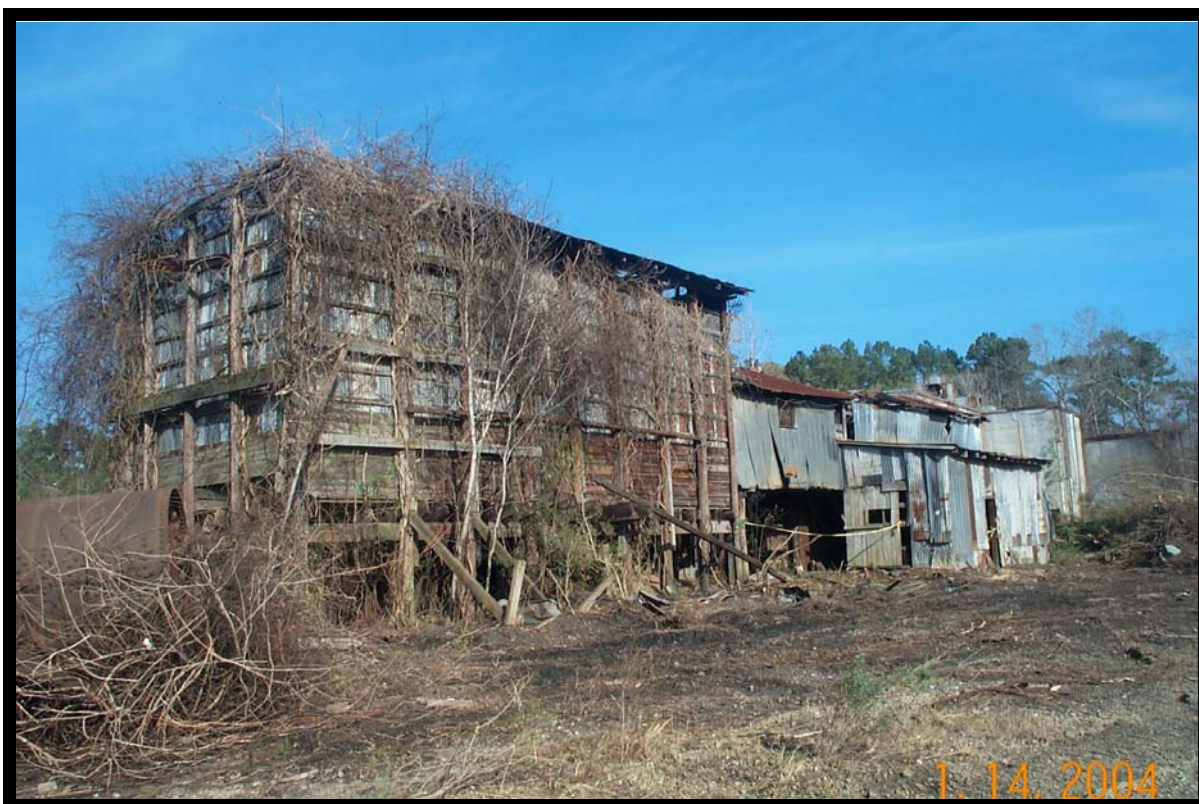
January 2004 - The former wood treating process area before construction of the remedy begins.
