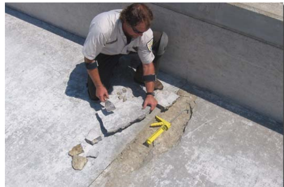
John Johnston prepares a crumbling concrete raceway floor for repair. -Photo by Wayne Talo
