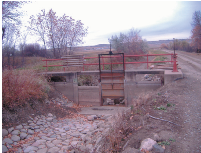
The end of delivery system site. The spill gate (to the right of the check) is being motorized and will be automated to maintain canal pool level within a target range.
