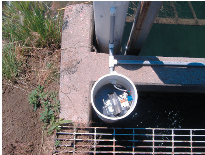
Upstream and downstream stilling wells retrofitted into the constant head orifice structure at the head of the 7.2 lateral at Angostura Irrigation District. A “homemade” float and pulley sensor is seen installed in the downstream 6-inch diameter well.
