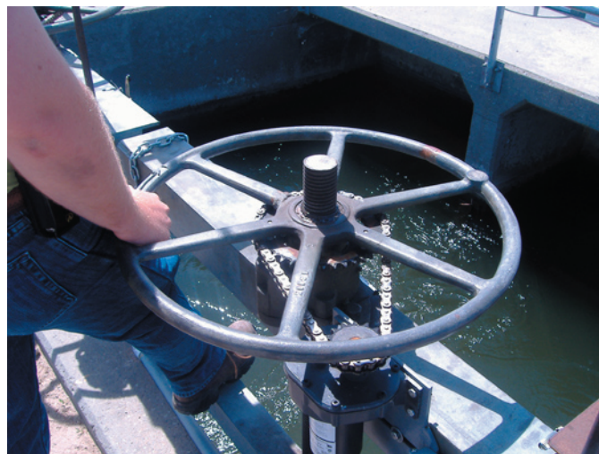
The motorization modifications on a gate at the Airport Lateral headworks at the Ainsworth Irrigation District. The chain drive system was installed by district personnel using methods jointly concocted by the district staff and WRRL researchers.
