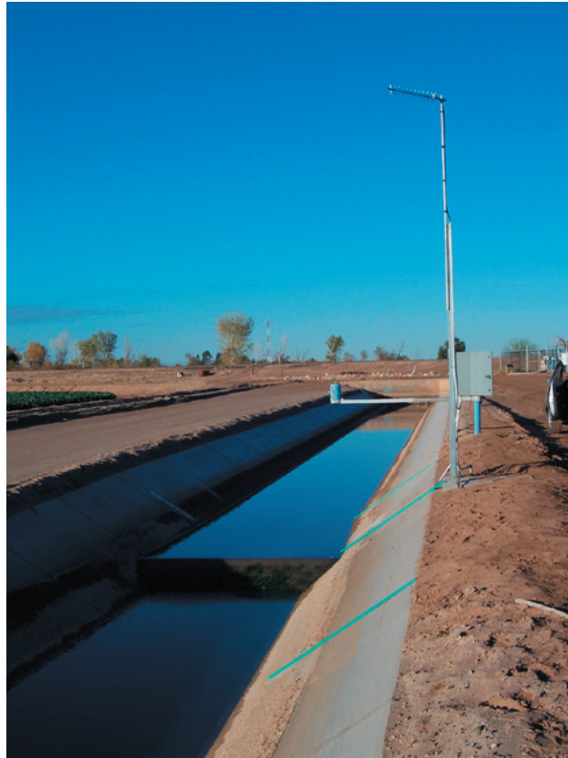
A view of a YCWUA flume looking upstream. Bubbler tubes for the level sensing system are installed underneath the green strips seen attached to the canal lining.
