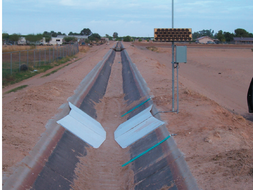
A new laterally contracted, long-throated flume that was installed with the submerged measurement bubbler system at the Unit B Irrigation District. A flume had not previously been installed at this site due to submergence concerns.
