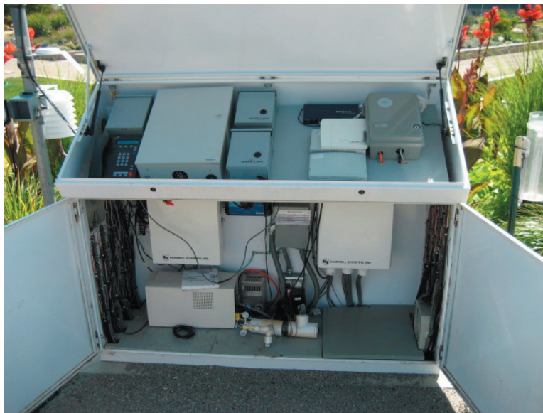
Cabinet containing data logging equipment from sensors.
