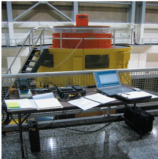
174-MVA generator at Glen Canyon Powerplant, on which generator acceptance tests were performed and used to test the new method for calculating generator leakage reactance. A TSC test instrumentation table to collect data for the tests is shown as well.
