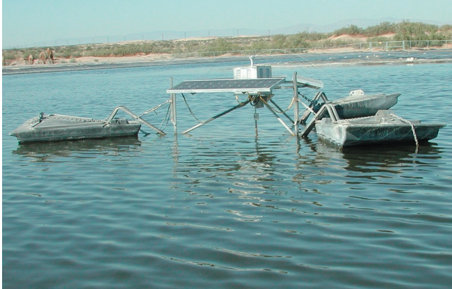
A SolarBee® pond circulator
